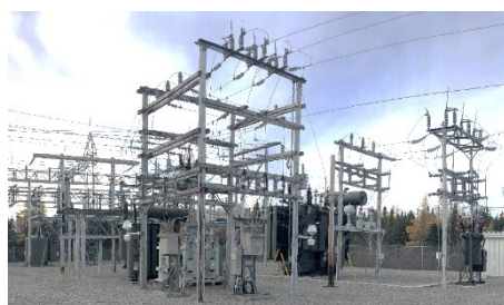
Gambo Substation in Central Newfoundland and Labrador.
