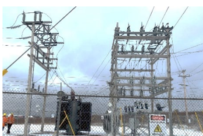
Old Perlican Substation in Avalon.
