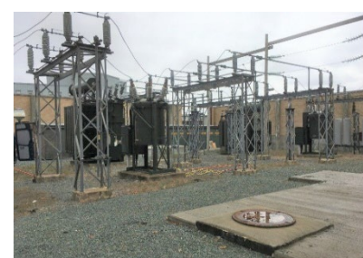
Memorial Substation in St. John’s.
