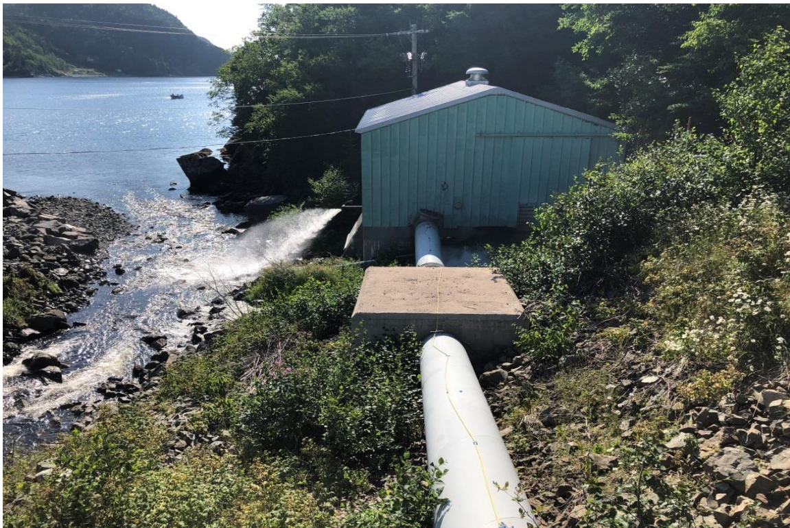
Figure 5: Snook's Arm Generating Station
