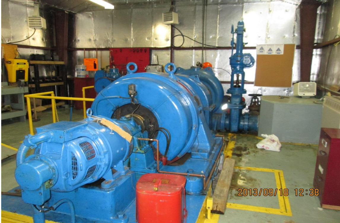
Figure 10: Venams Bight Hydraulic Generating Unit
