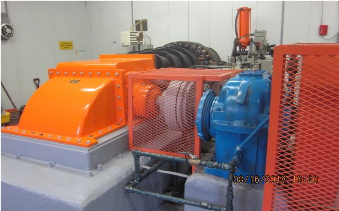
Figure 3: Roddickton Generating Unit
