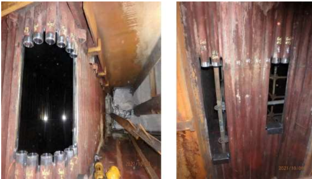
Figure 4: Portion of Removed Waterwall Tube Section on Unit 3 Boiler
