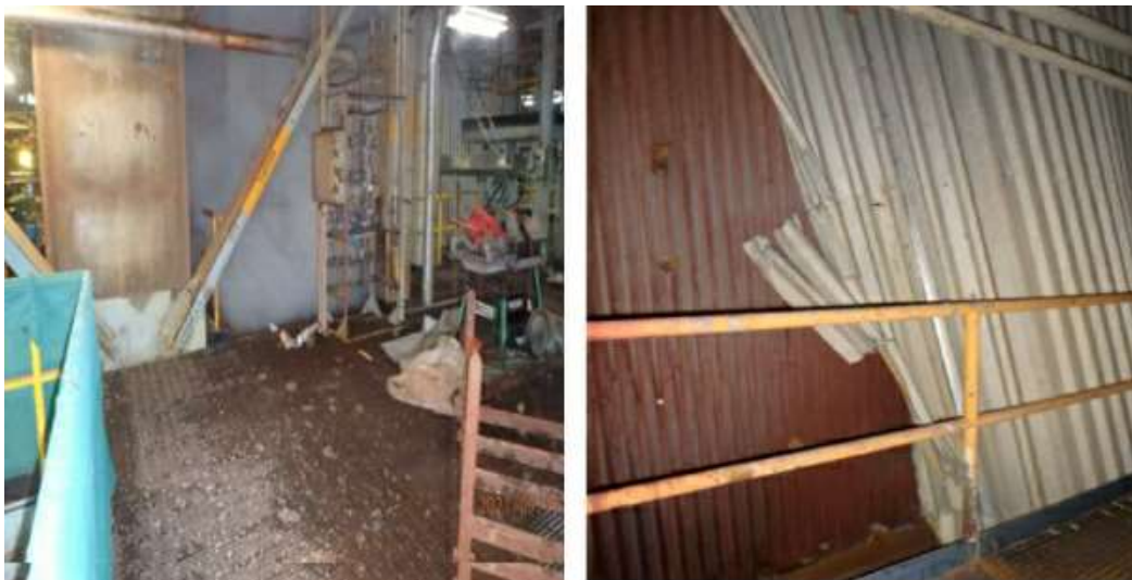
Figure 2: Debris, Released Steam and Cladding Damage on Unit 3 Boiler
