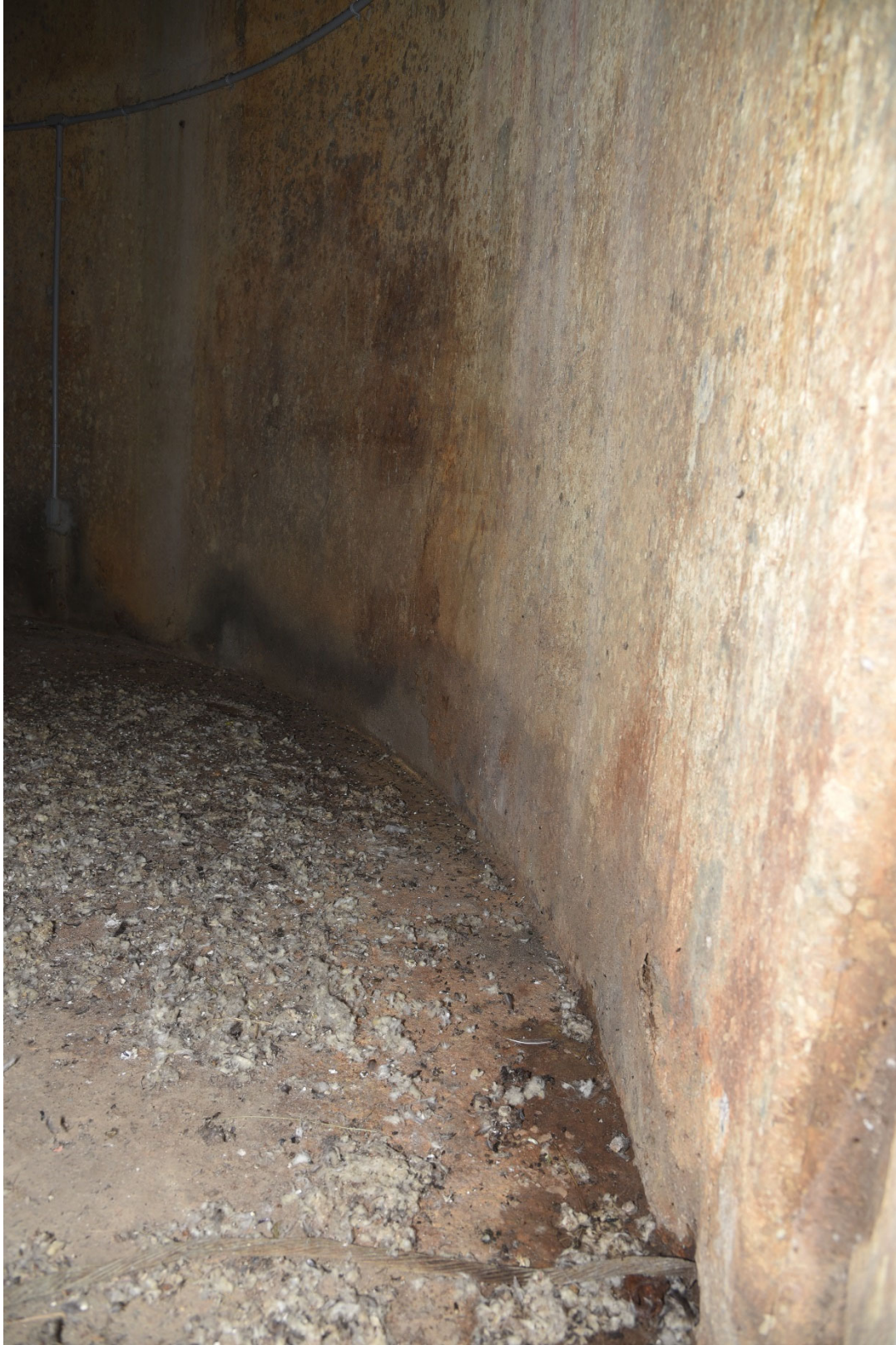
Exhaust Stack No. 2 Internal View of the Concrete Shell to Foundation Connection
