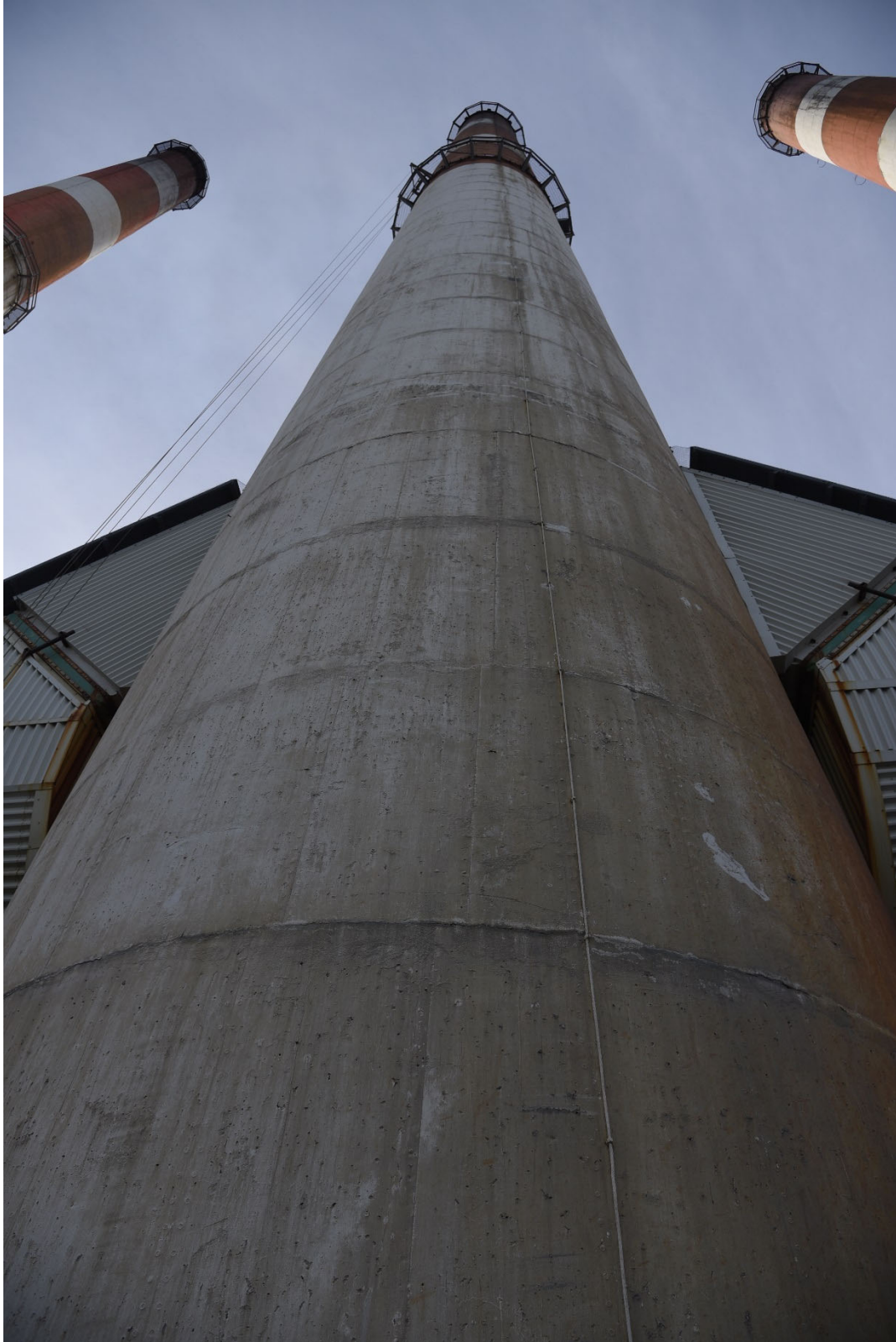
View of Exhaust Stack No. 2 Looking Upward from East Side. – Circumferential Construction Joints are Visible
