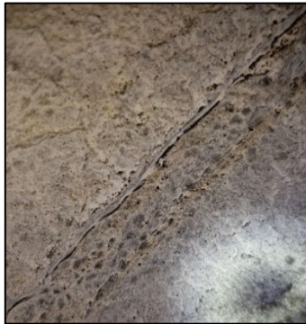
Figure 3-1: Sample of Deteriorated Longitudinal Weld Seam
