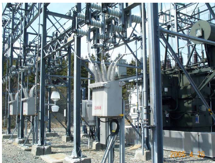
Foundation damage at Clarkes Pond Substation
