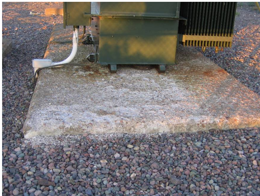
Foundation damage Garnish Substation
