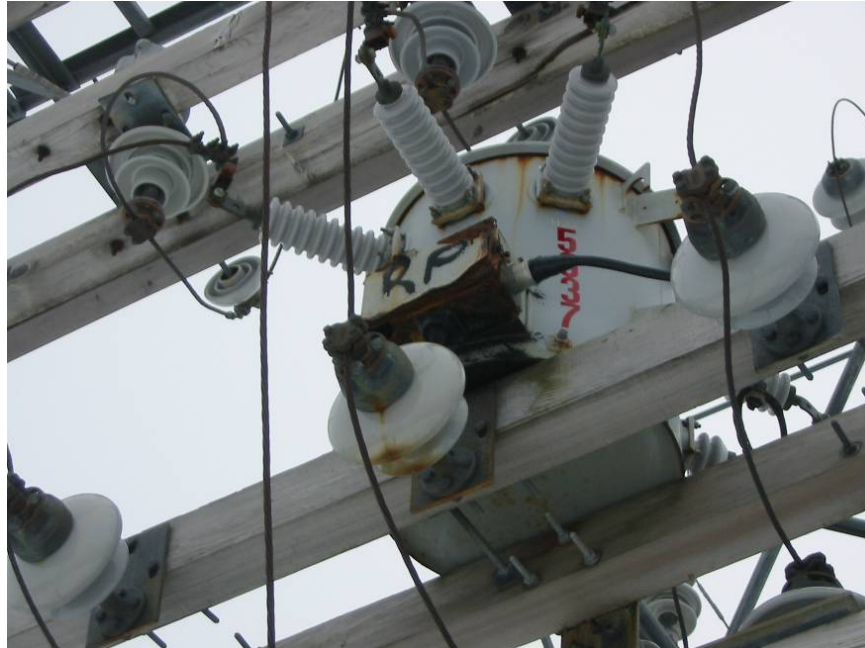
Corrosion damage Garnish Substation
