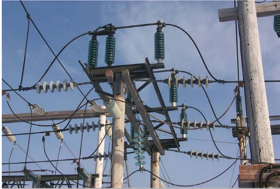
Bus Tie Switch Bypassed Goulds Substation
