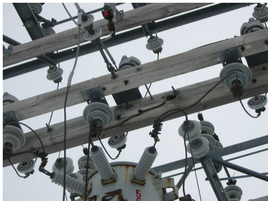
Cracked crossarm Garnish Substation
