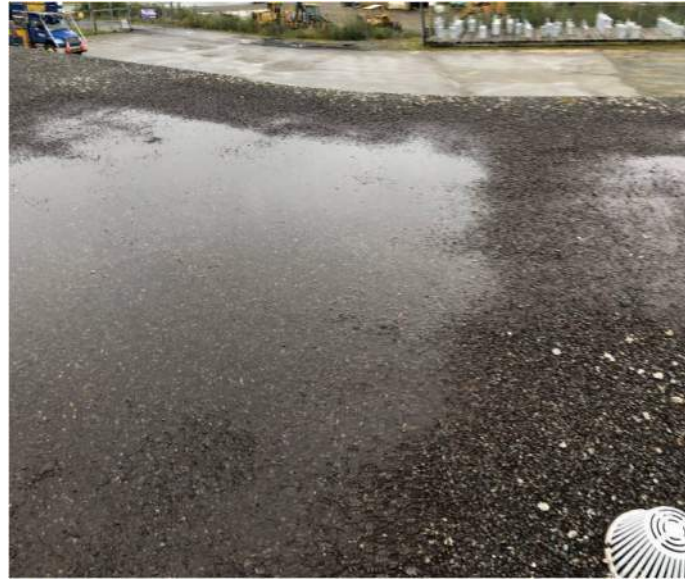
PHOTO 18: STAGGING AREA BUILT-UP ROOF WITH WATER PONDING.
