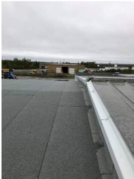
PHOTO 13: TRANSITION WALL BETWEEN THE MAIN BUILDING ROOF AND STORAGE AREA METAL ROOF.
