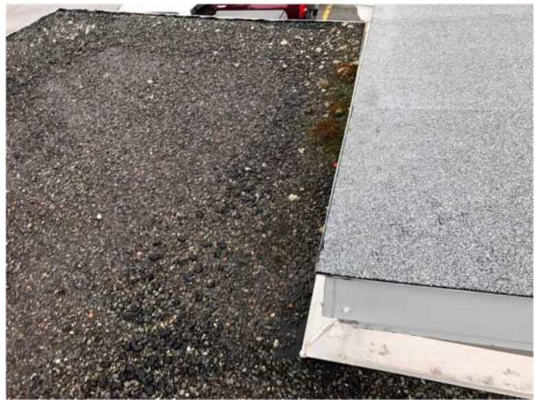
PHOTO 6: VESTIBULE BUILT-UP ROOF WITH LOCALIZED MOSS AND VEGETATION GROWTH.
