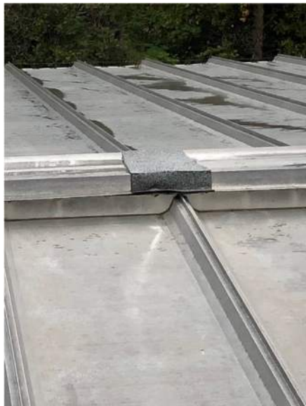
PHOTO 15: SEAM OF RIDGE FLASHING OF THE PITCHED STANDING SEAM ROOF COVERED WITH A STRIP OF MODIFIED BITUMEN MEMBRANE.
