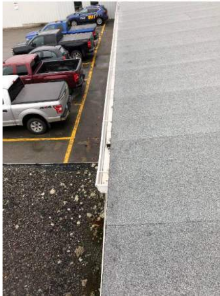
PHOTO 9: EAVES THROUGH AT GABLE SINGLE-PLY MODIFIED BITUMEN ROOF.
