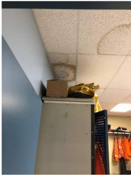
PHOTO 5: REPORTED LEAKS IN THE LINE PERSON DRYROOM.
