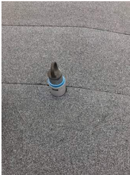
PHOTO 11: ROOF ANCHOR INSTALLED ON THE SINGLE-PLY MODIFIED BITUMEN MEMBRANED ROOF.
