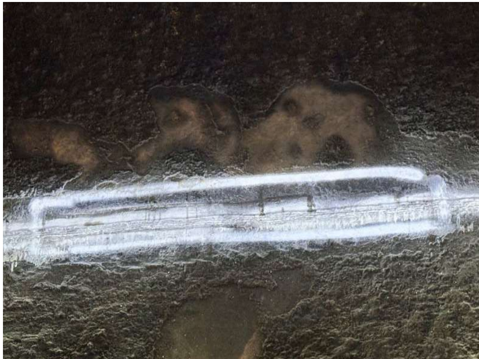
Photo 14 Close-up of intermittent weld indication at Can 17S
