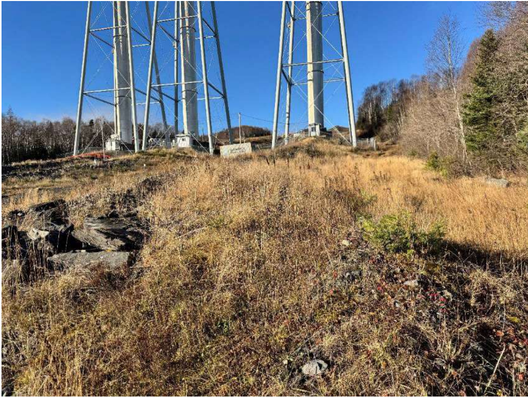
Photo 7 Vegetation impeding visual access to exterior of penstock
