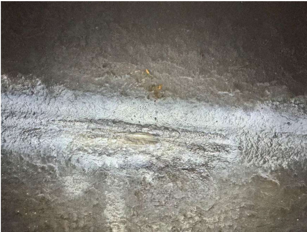
Photo 27 Close-up of weld indication removed with grinding at Can 353N
