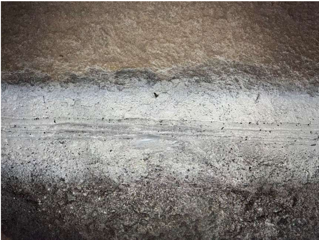
Photo 25 Close-up of weld indication removed with grinding at Can 322N
