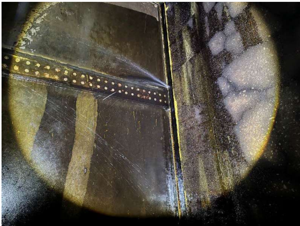
Photo 4 Leakage through seal on left side of gate
