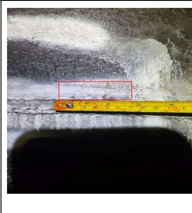
Figure 2. Can 17 South - Indication #1 - Intermittent Indication Noted
