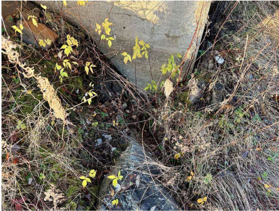
Photo 42 Condition of concrete at left side of downstream face of surge tank concrete base
