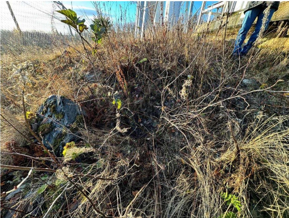
Photo 40 Sinkhole downstream of surge tank concrete base
