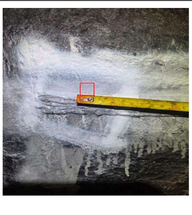
Figure 3. Can 17 South - Indication #2
