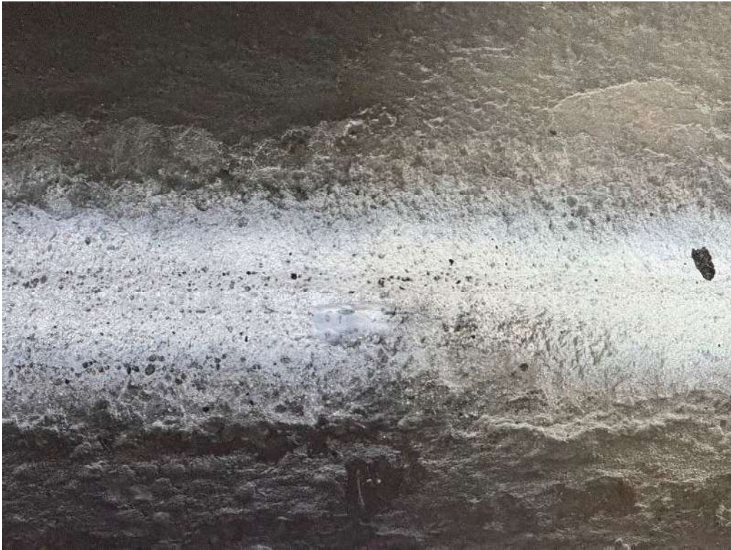
Photo 23 Close-up of weld indication removed with grinding at Can 273N
