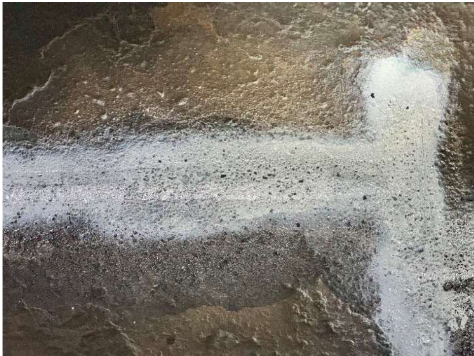
Photo 24 Close-up of weld indication removed with grinding at Can 303N
