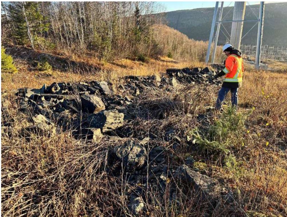
Photo 6 Brush impeding access to exterior of penstock
