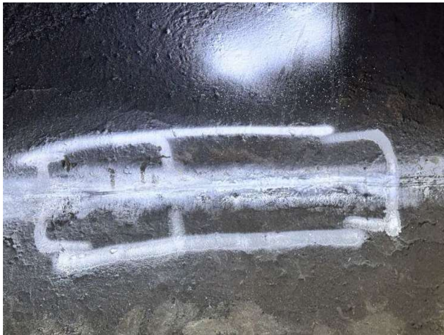
Photo 18 Close-up of intermittent weld indication at Can 67S
