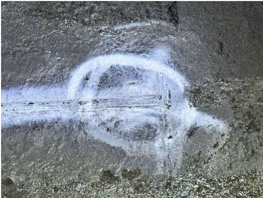
Photo 20 Close-up of intermittent weld indication at Can 102S
