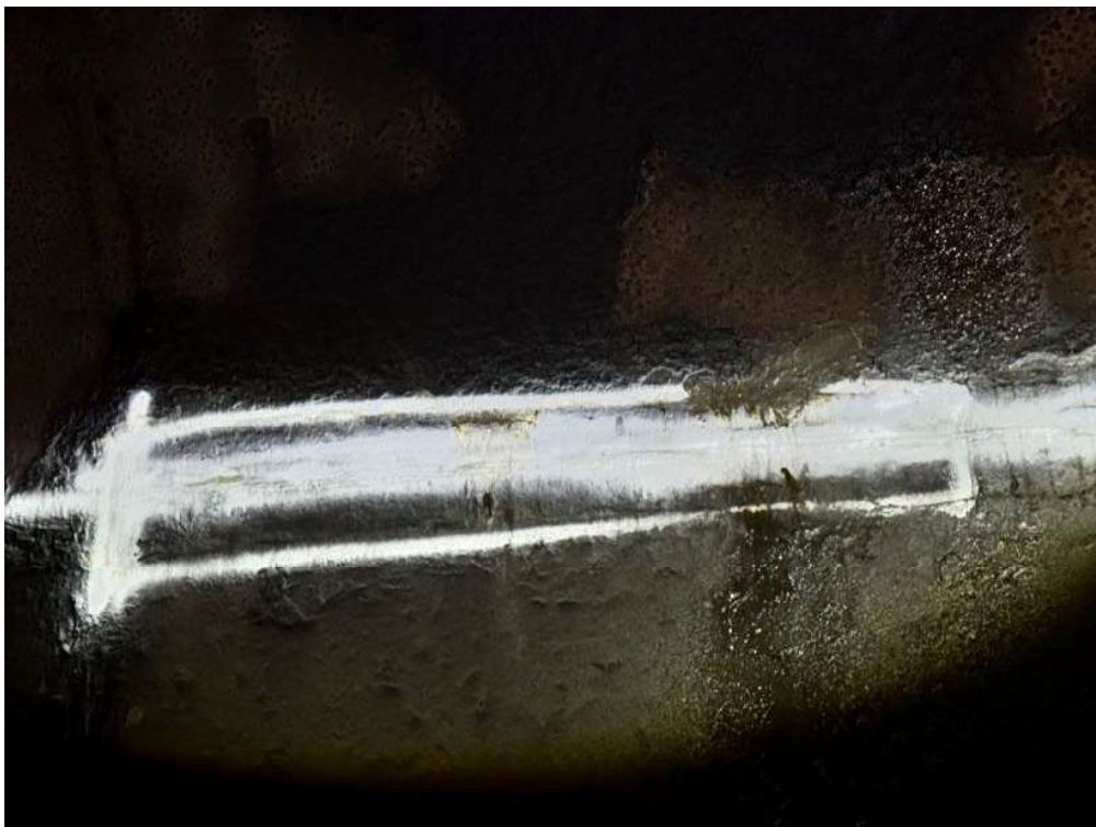
Photo 16 Close-up of intermittent weld indication at Can 35N
