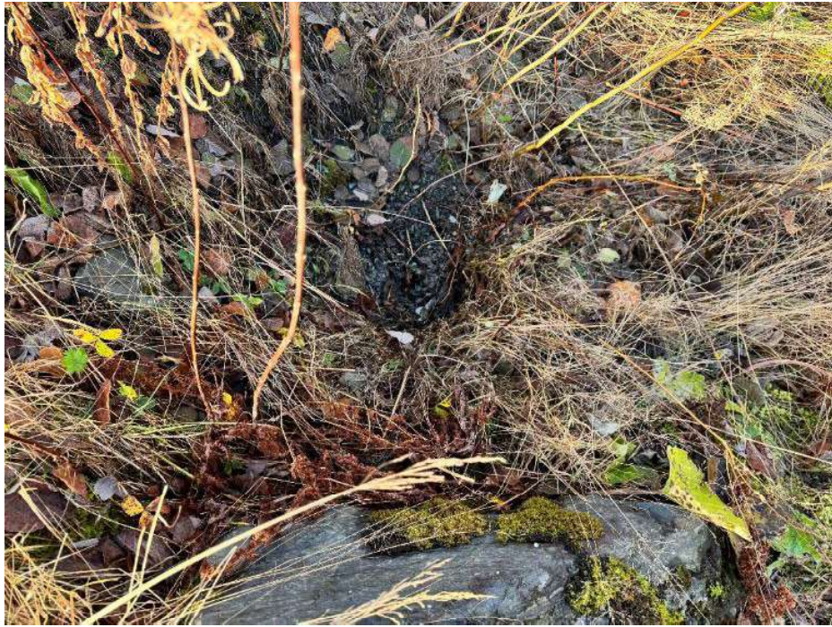
Photo 41 Sinkhole downstream of surge tank concrete base
