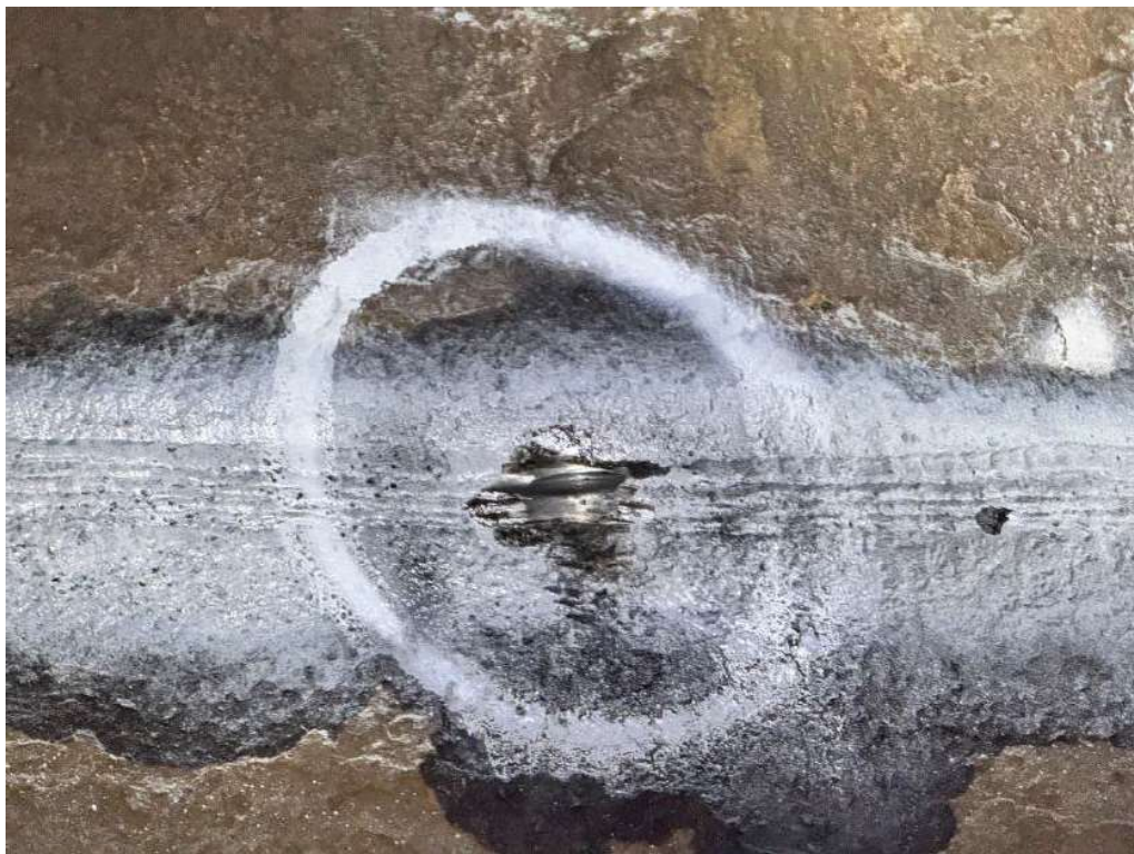
Photo 26 Close-up of weld indication at Can 332N
