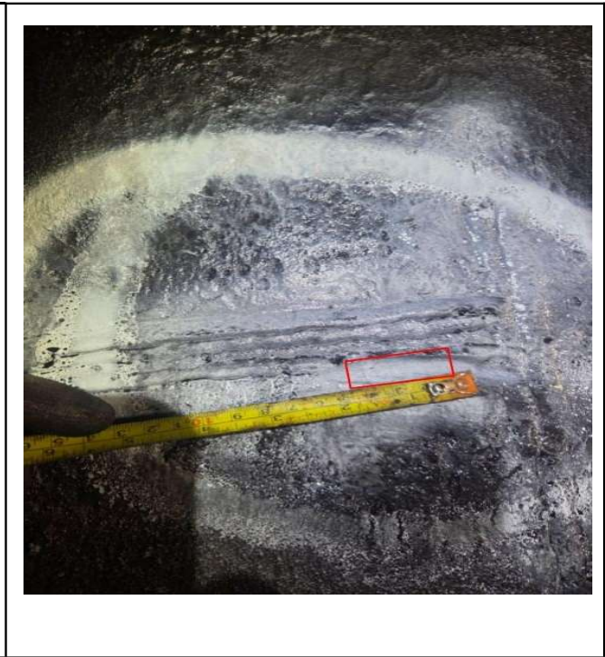
Figure 13. Can 102 South - Indication #7
