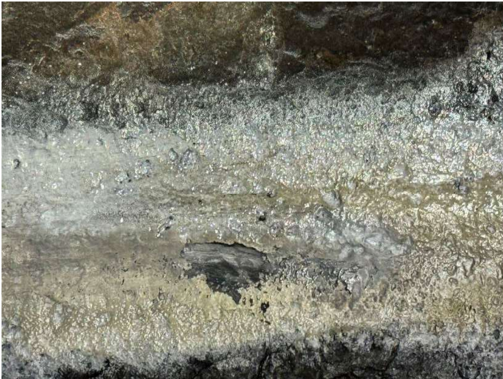
Photo 22 Close-up of weld indication at Can 263S
