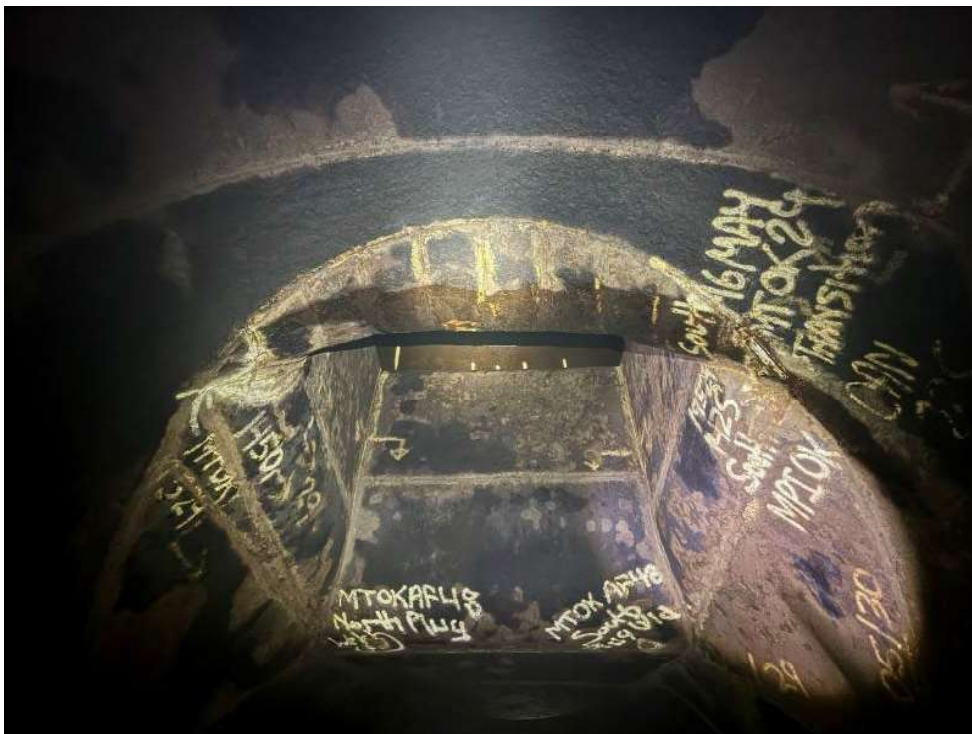
Photo 28 Leakage observed at upstream side of surge tank transition
