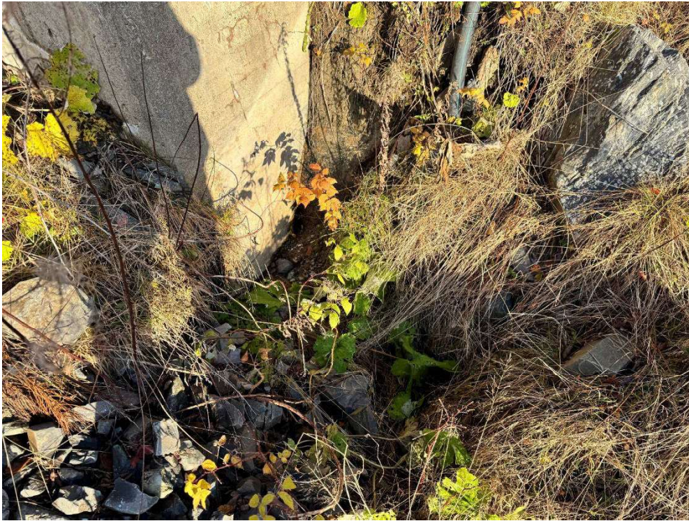
Photo 39 Condition of concrete at right side of downstream face of surge tank concrete base
