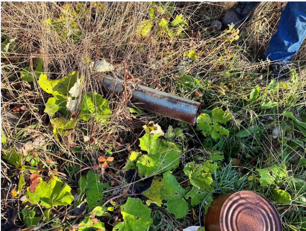
Photo 38 Condition of drainage pipe directly downstream of surge tank concrete base
