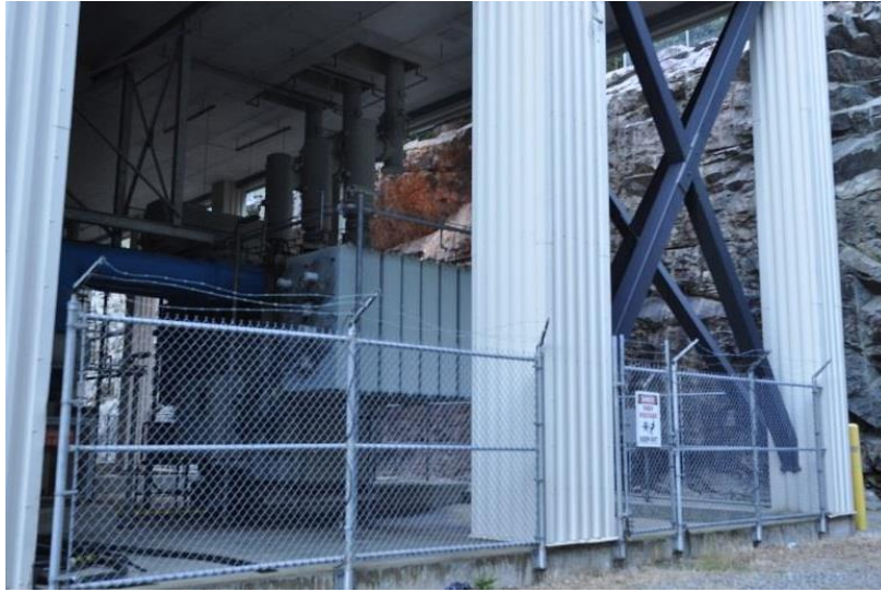
Figure 2: Chain-Link Fencing around Exterior Transformers
