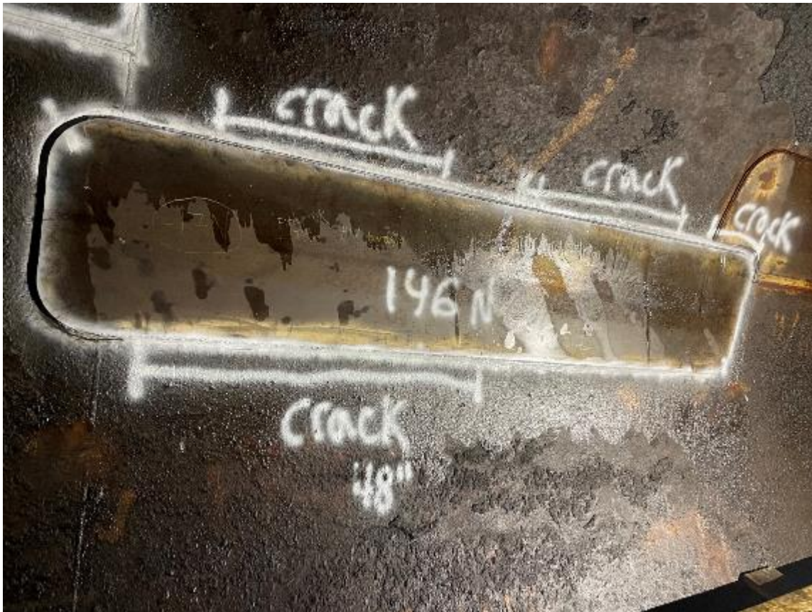
PHOTO 5 CRACKING AROUND WELD REINFORCING PLATE, CAN 146 NORTH SIDE
