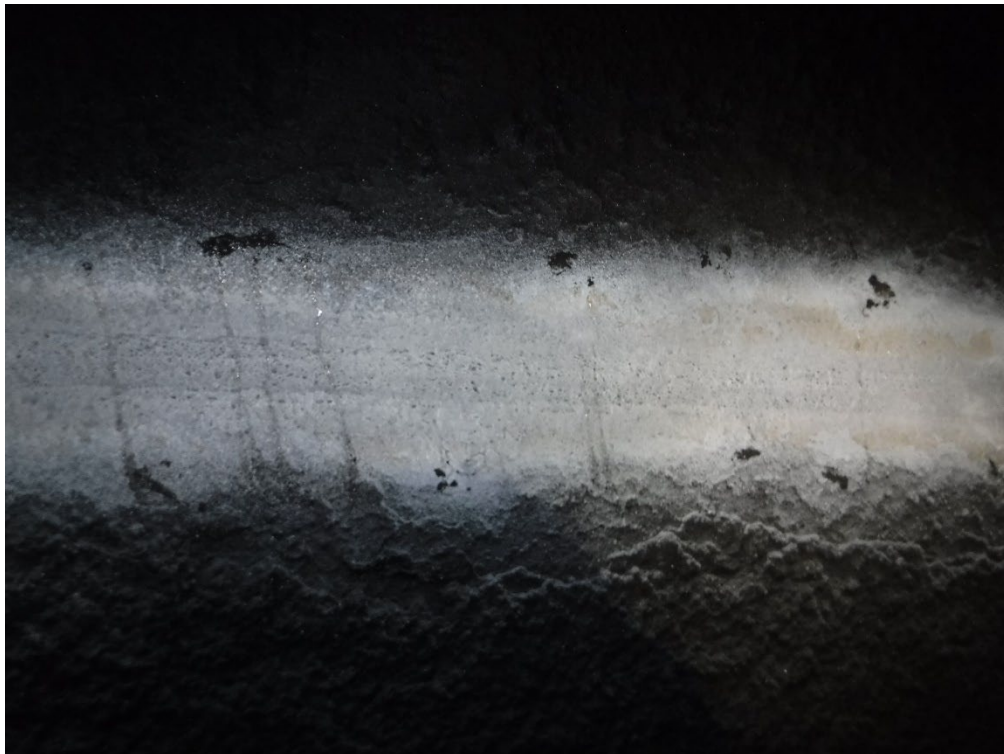
Photo 10 Original weld not tested previously; Can 268; Typical Condition
