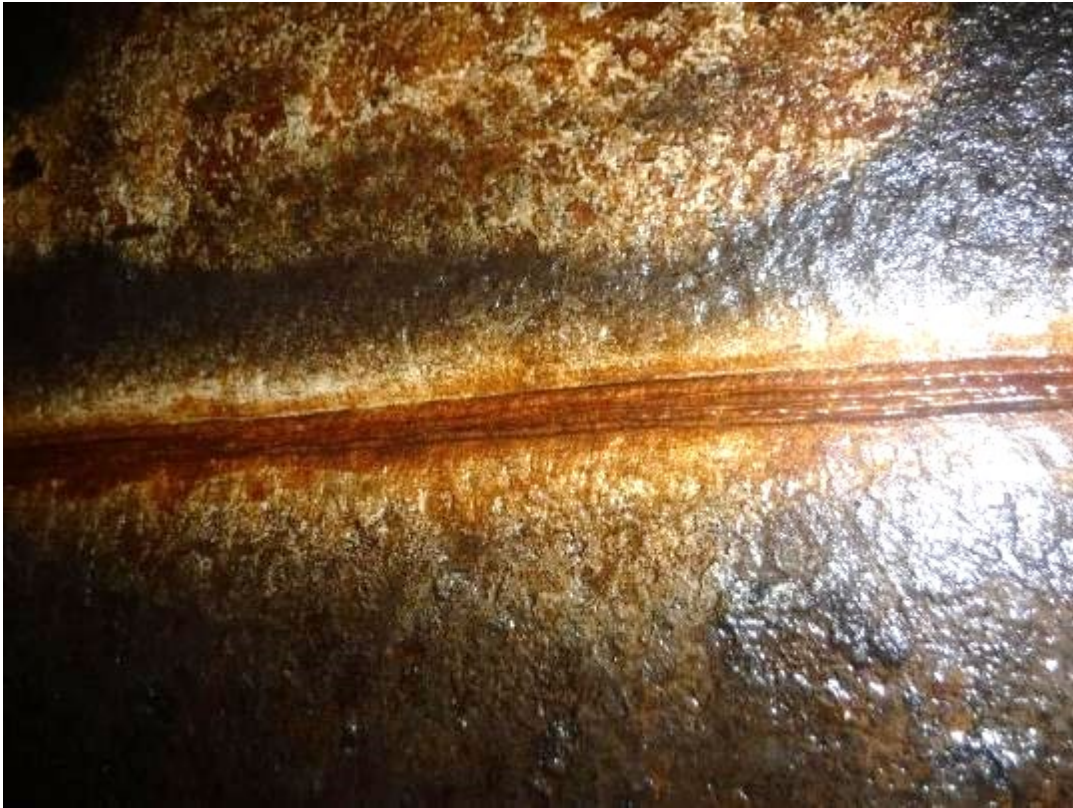
Photo 7 Typical repaired weld not tested this year
