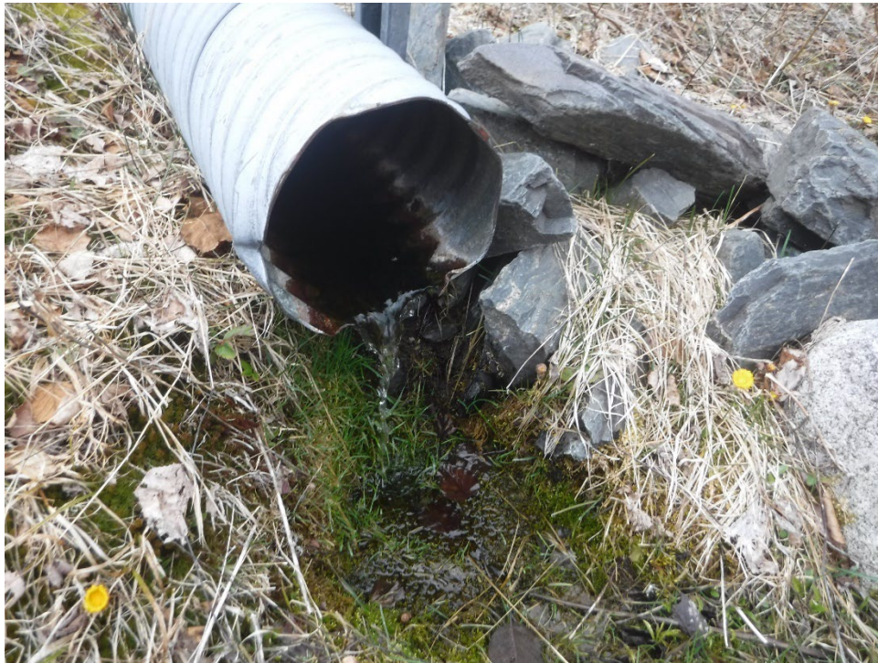
Photo 17 Flow Pipe, FP 3
