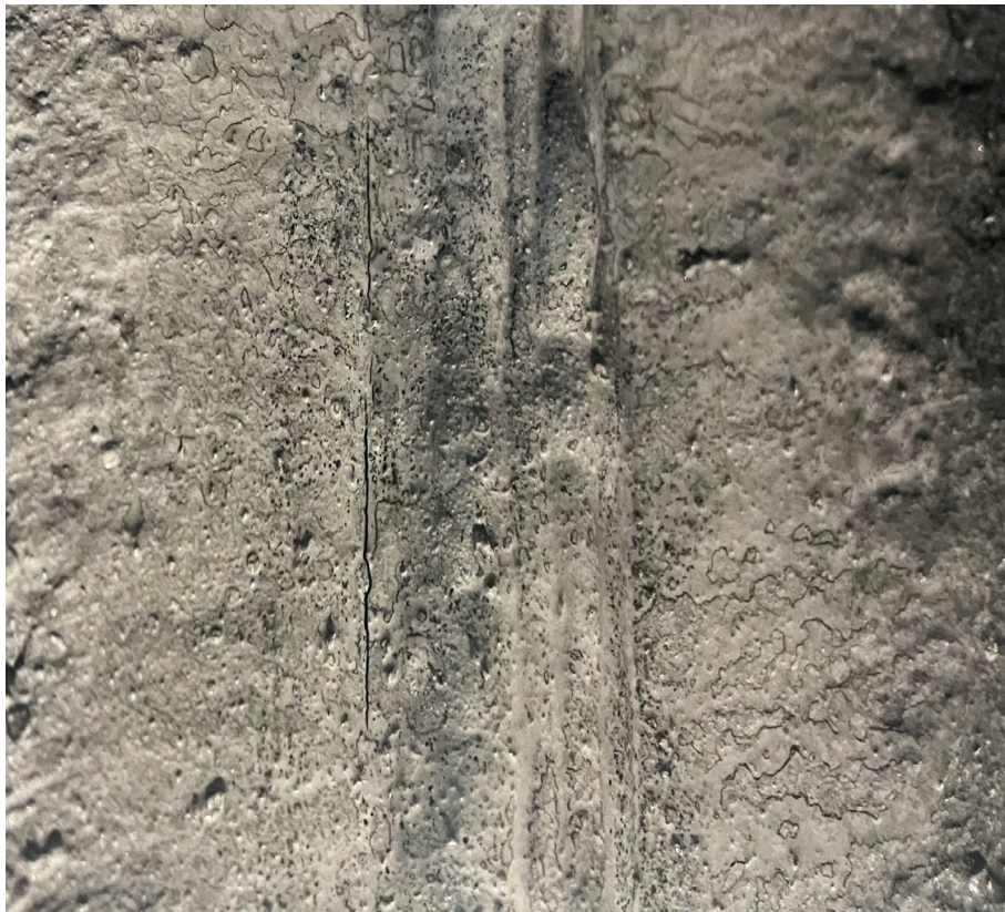
PHOTO 4 CRACK ABOVE LONGITUDINAL WELD NORTH SIDE CAN 126
