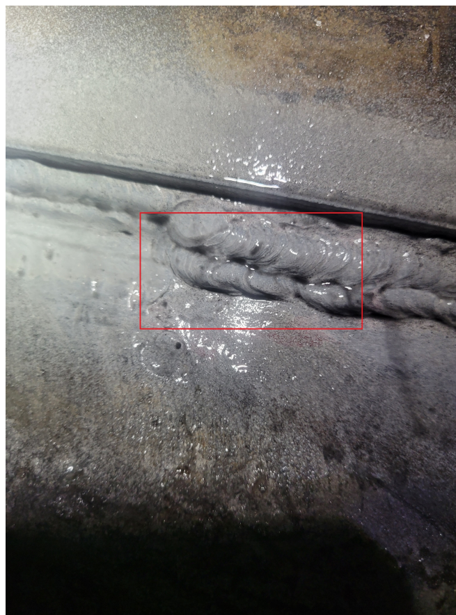
Figure 6. Can 146N - Indication Noted
