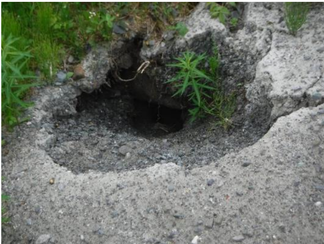
Photo 40 Sink hole downstream of penstock 3 surge tank
