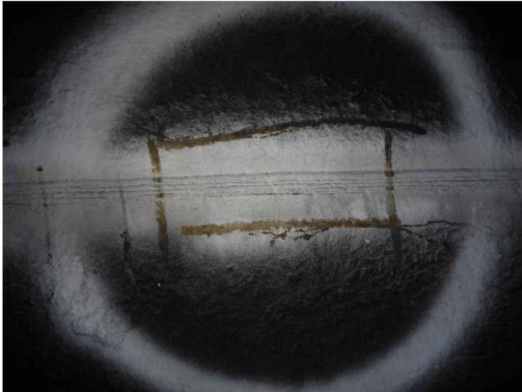
PHOTO 11 INDICATION OF ISSUE CAN 111 WELD NEAR SPRING LINE
