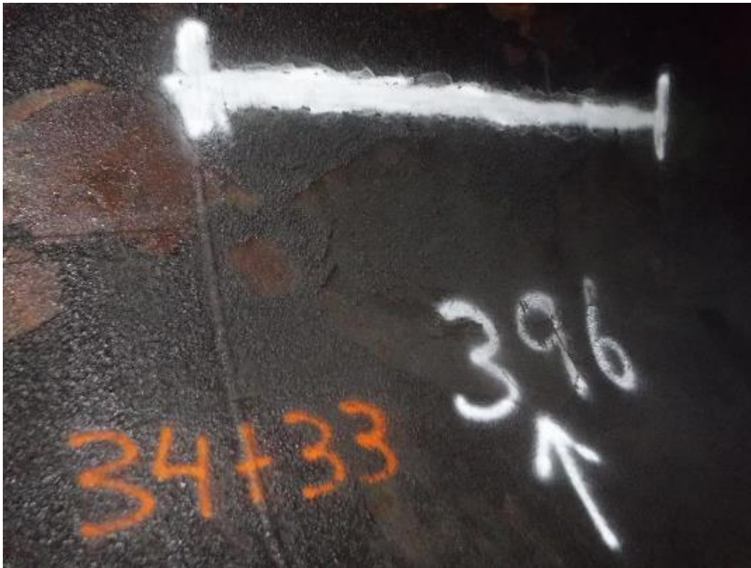
Photo 19 Tested weld Can 396
