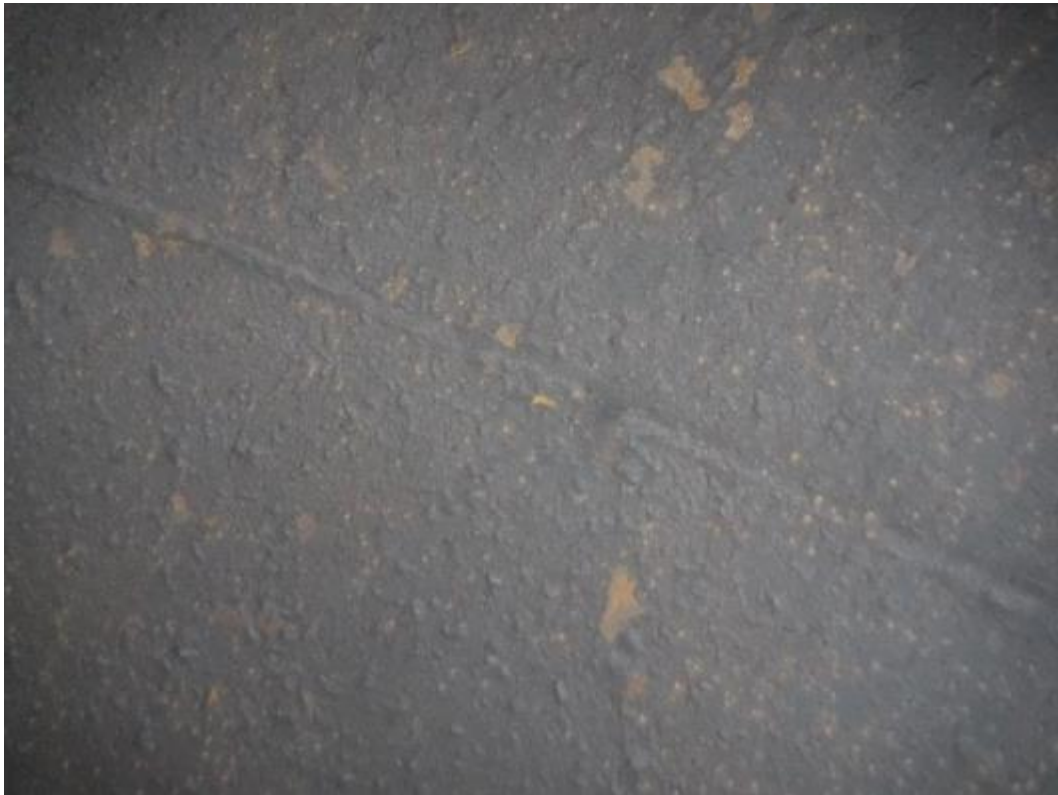
Photo 24 Surface conditions and original weld covered in organics Can 352
