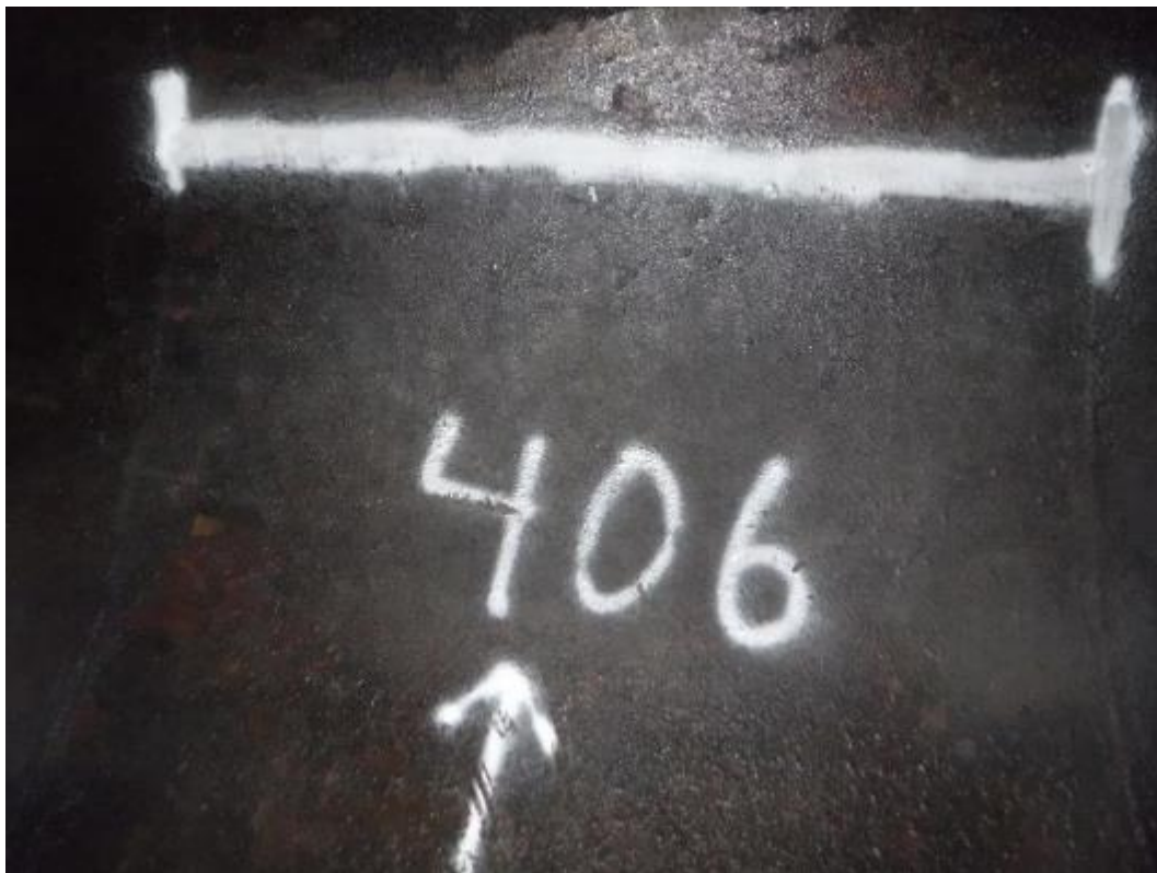
Photo 20 Tested weld Can 406
