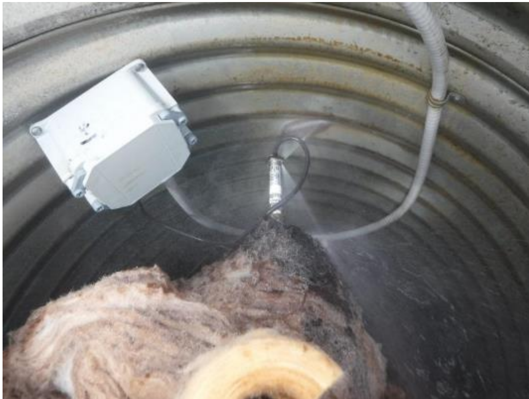
Photo 39 Leaking pressure transducer Penstock 2 upstream Station 900m
