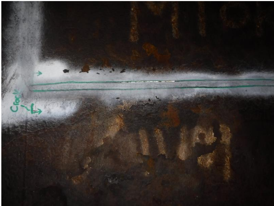
PHOTO 6 CRACKED WELD RIGHT SIDE OF CAN 106 NEAR SPRING LINE
