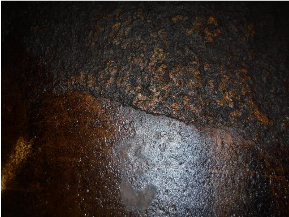
PHOTO 3 OLD ORGANIC GROWTH ON INSIDE OF PENSTOCK
