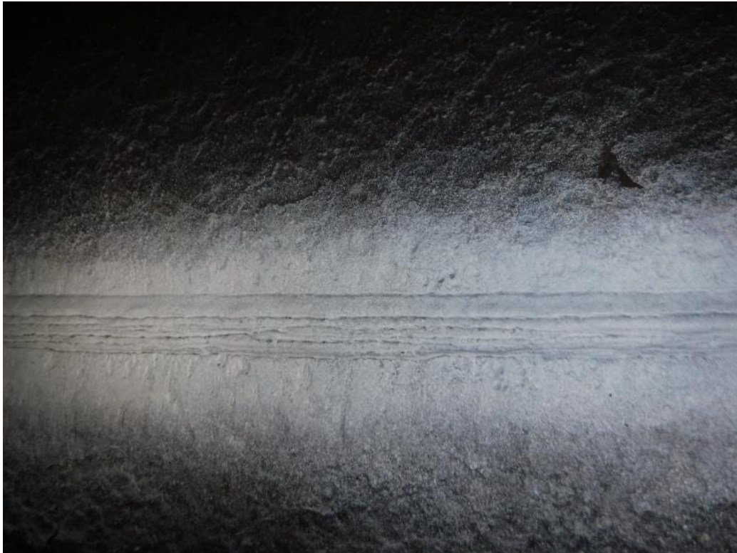
PHOTO 17 TEST OF PREVIOUSLY REPAIRED WELD CAN 123
