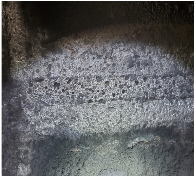
Figure 1. Can 336 - Pitting in Right Horizontal Weld Pre-Inspection (12" Section)
