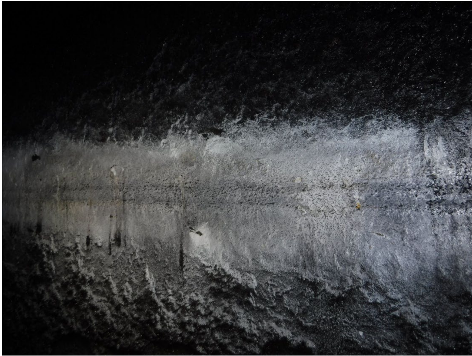
Photo 11 Original weld not tested previously; Can 188; Typical Condition
