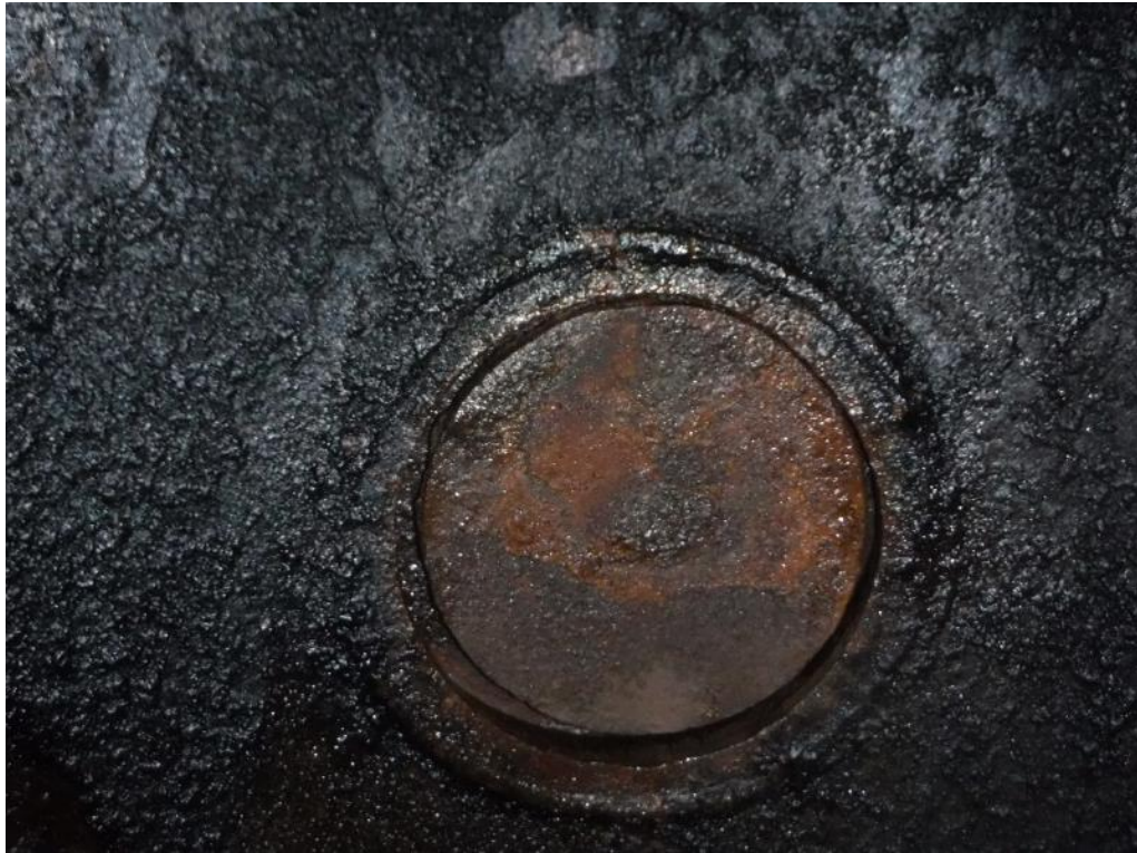
PHOTO 21 MANHOLE 3 NOT OPENED.
