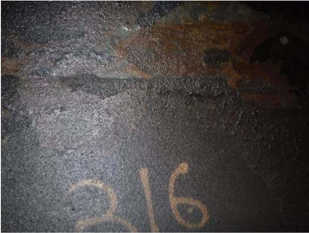
Photo 23 Surface conditions and original weld covered in organics Can 316
