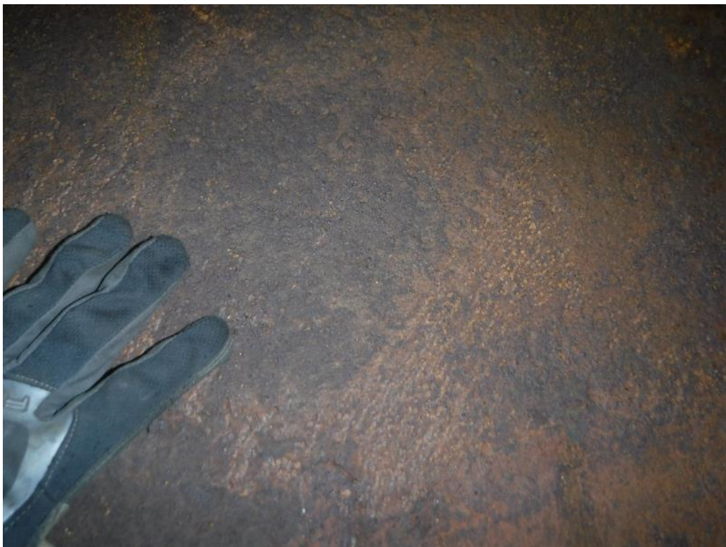
PHOTO 18 SURFACE CORROSION CAN 320 – LESS PITTING THAN HIGHER IN PENSTOCK
