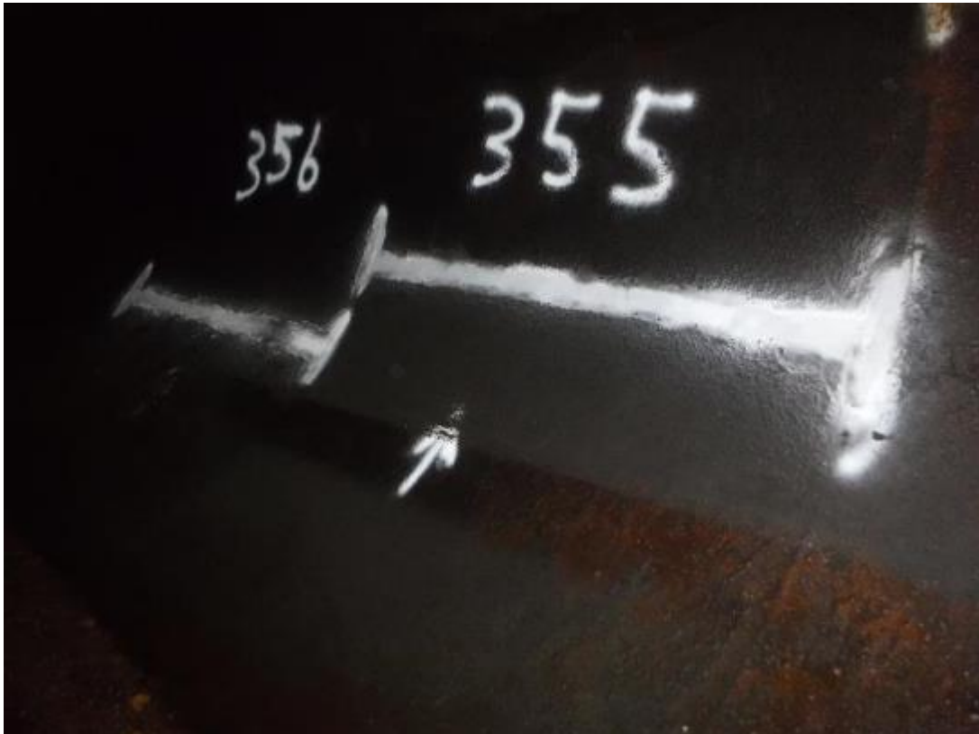
Photo 18 Tested weld Can 355
