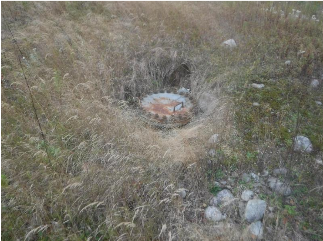
PHOTO 33 MANHOLE 3 AT TOP OF STEEP SLOPE
