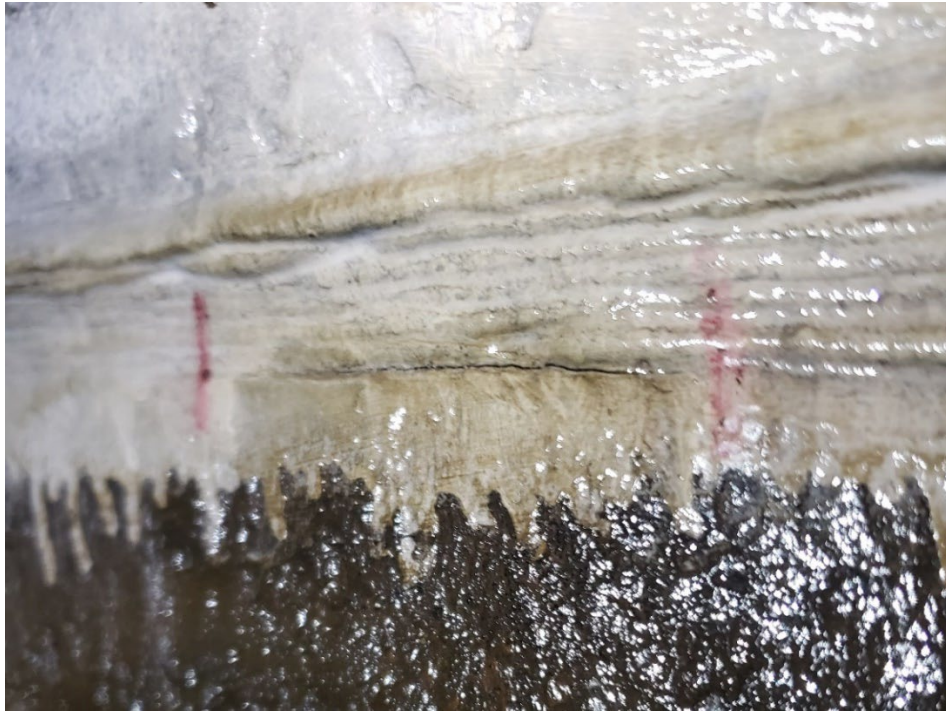
Photo 13 Longitudinal Weld Crack Can 145 North Side
