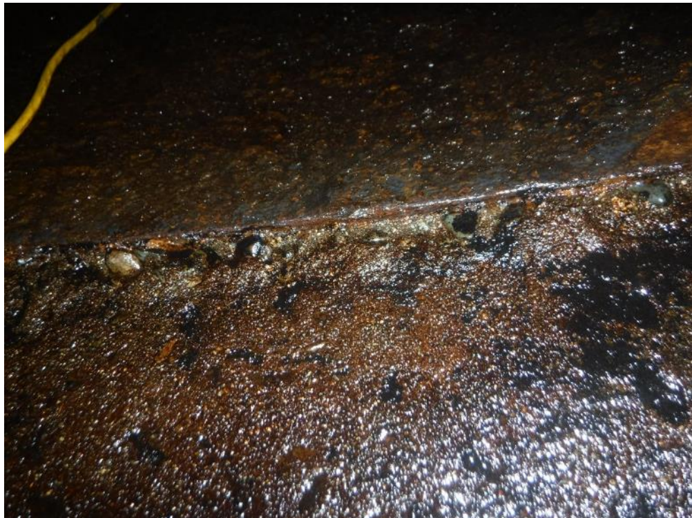
PHOTO 2 CONCRETE DETERIORATION AT CONCRETE TO STEEL TRANSITION
