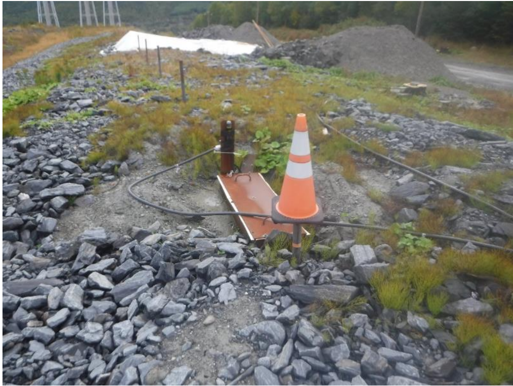
PHOTO 27 PIEZOMETER LOCATION JUST UPSTREAM OF CRACK LOCATION
