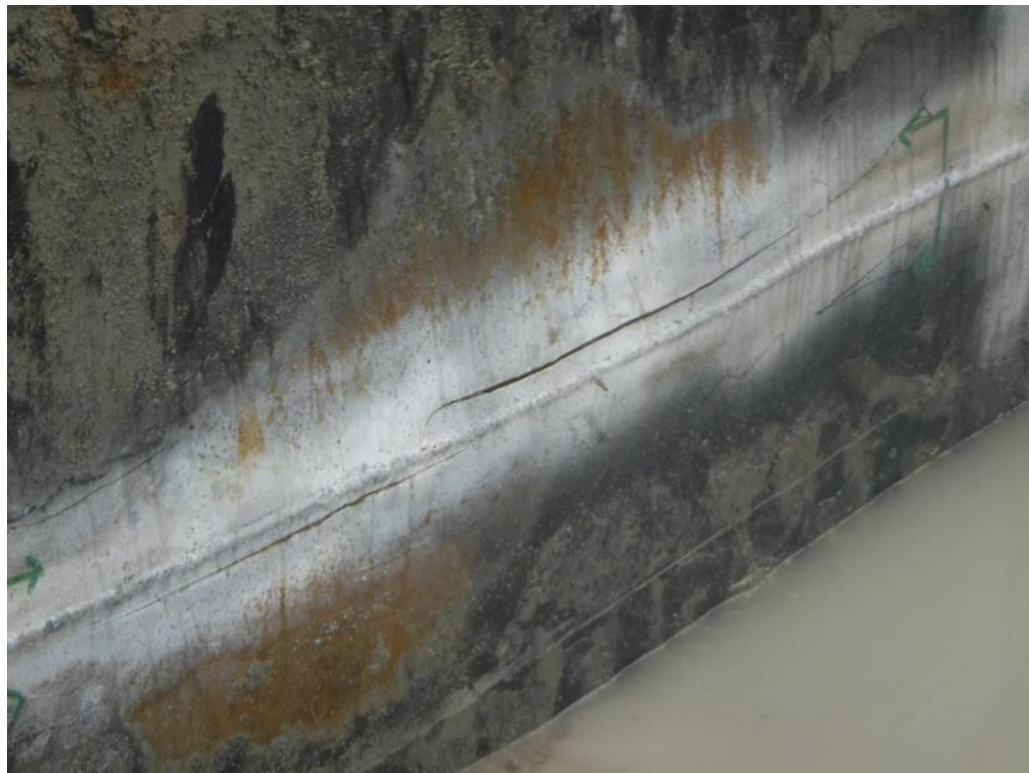
PHOTO 8 CRACKED WELD FROM OUTSIDE RIGHT SIDE OF CAN 106
