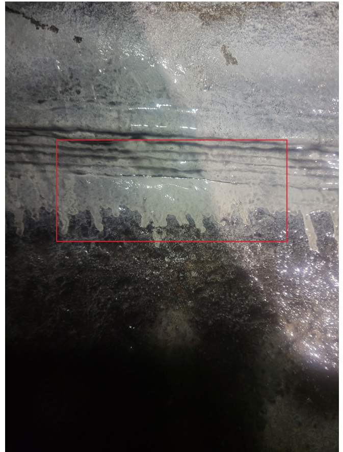
Figure 6. Can 145N - 3" Crack Indication Noted *Refer To Report 22-318 For Repair
