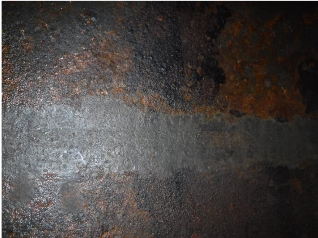
PHOTO 19 SURFACE SCRAPED DOWN TO SHOW LIGHT PITTING
