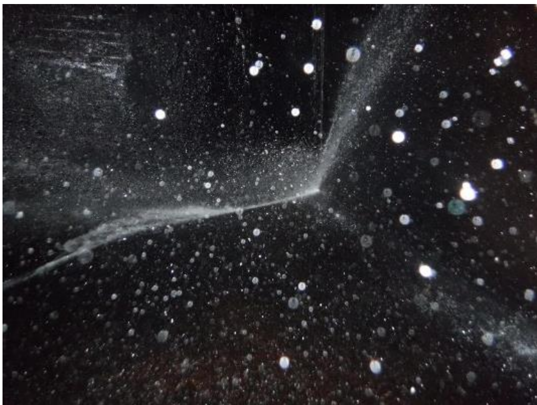
Photo 2 Leakage Bottom Right Corner of Gate
