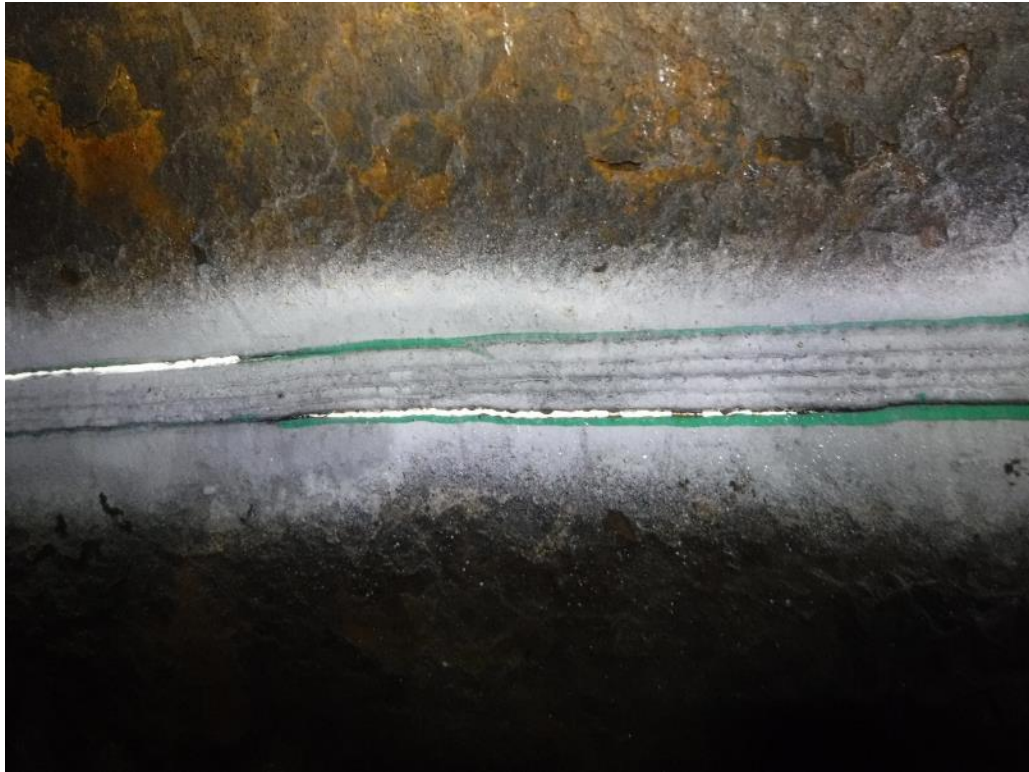
PHOTO 7 CRACKED WELD RIGHT SIDE OF CAN 106 NEAR SPRING LINE
