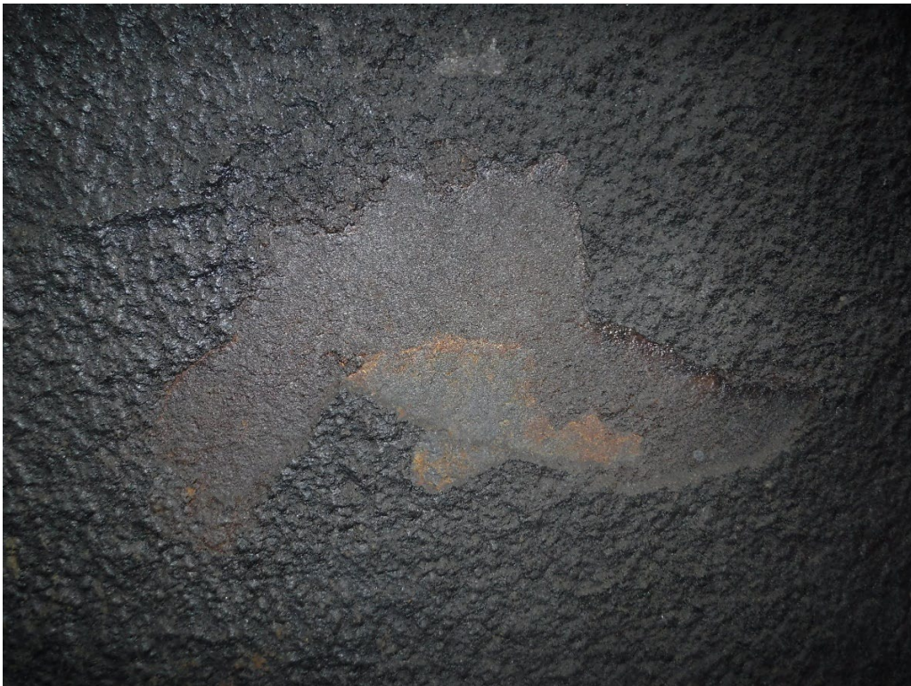
Photo 4 Organic Layer with Steel Beneath
