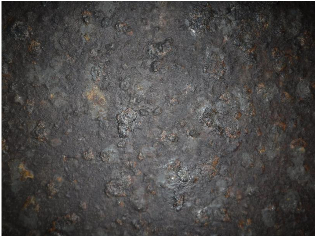
PHOTO 20 SURFACE CORROSION AND FLAKING CAN 200
