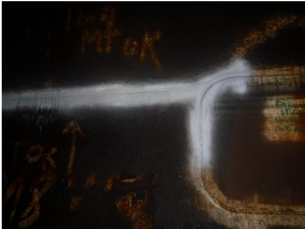
PHOTO 16 WELD TEST INCLUDED PART OF DOUBLER PLATE WELD
