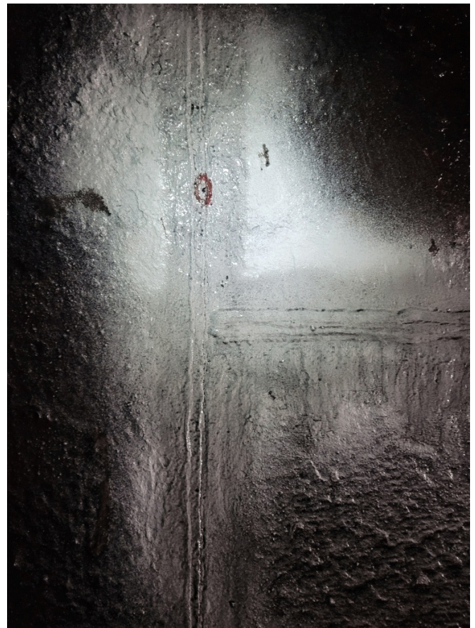
Figure 2. Can 98 North - Indication Noted
