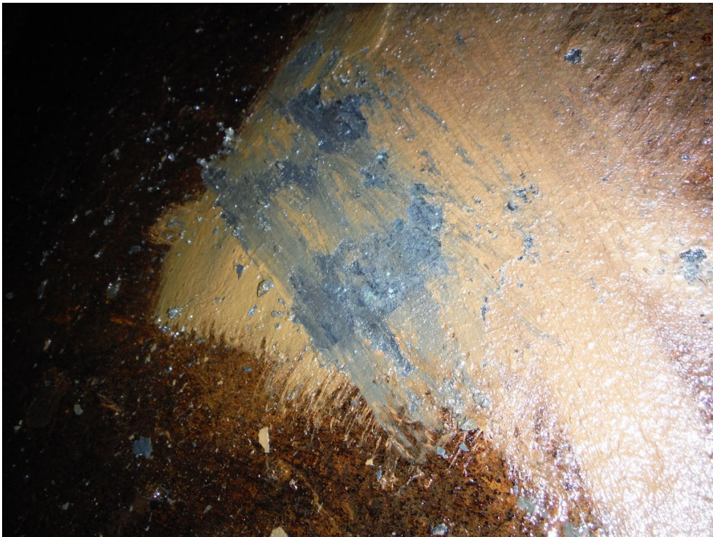
Photo 6 Plating lightly scraped; Shallow pitting and some section loss
