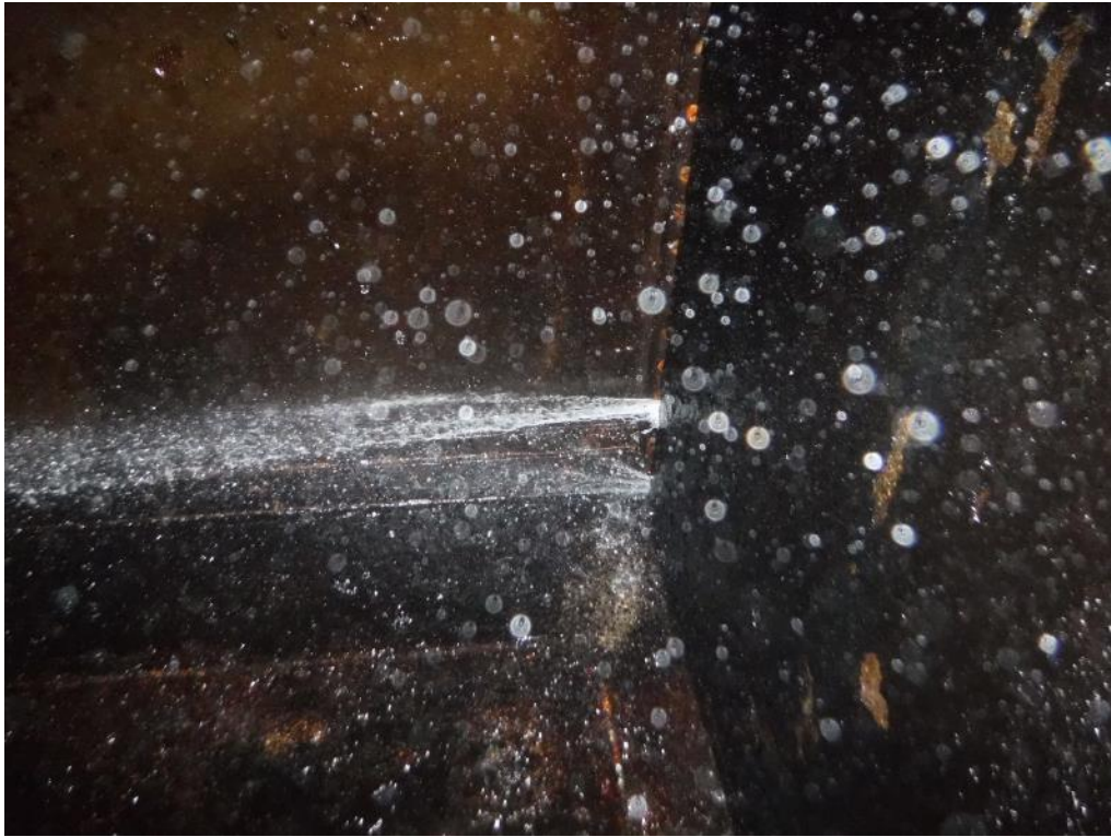
PHOTO 1 LEAK IN BOTTOM LEFT CORNER OF GATE
