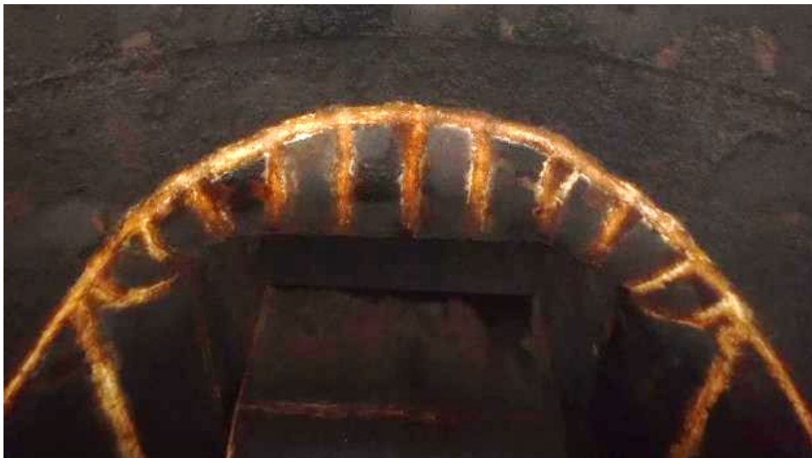
Photo 28 Surge tank transition welds
