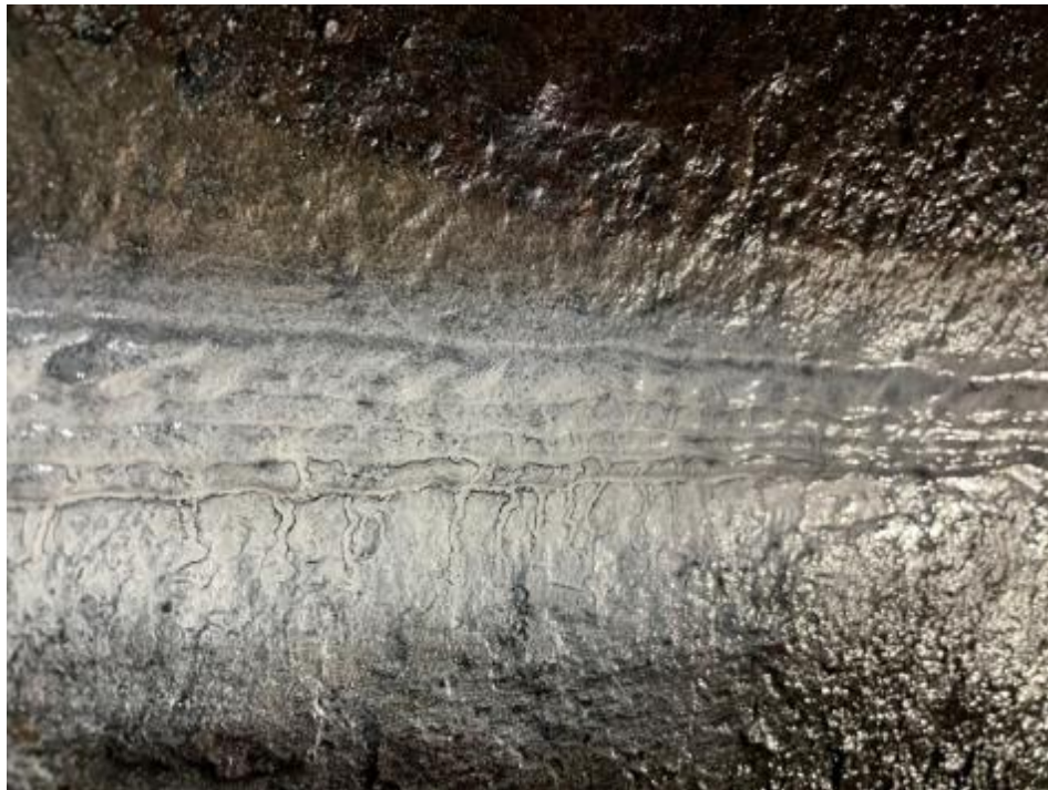
PHOTO 2 TYPICAL PREVIOUSLY REPAIRED WELD (CAN 12)
