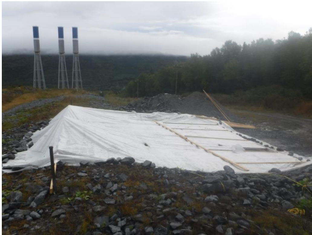
PHOTO 28 LOOKING DOWNSTREAM AT CRACK LOCATION COVERED IN TARP
