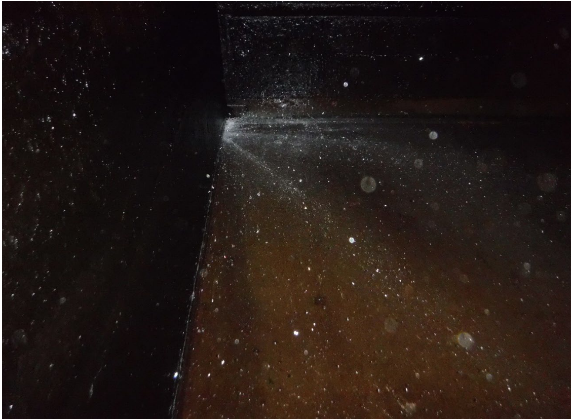
Photo 1 Leakage from Right Top Corner of gate
