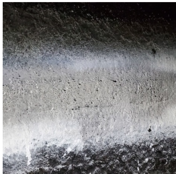
Figure 2. Can 336 - Pitting in Right Horizontal Weld Post-Inspection (12" Section)
