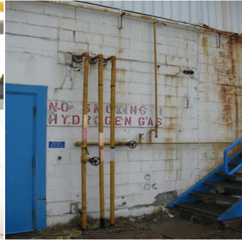
Figure 11-6 Hydrogen Lines into Powerhouse
