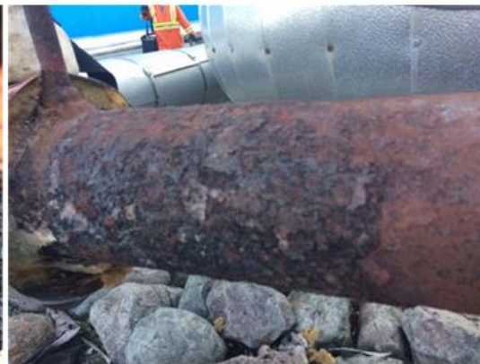
General corrosion noted prior to pre-cleaning
