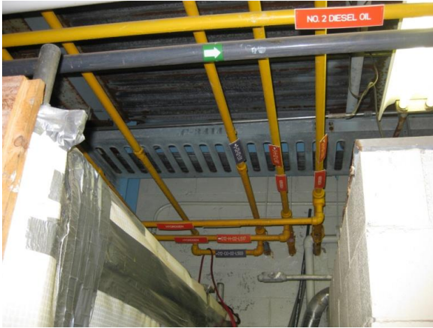
Figure 11-5 Hydrogen Lines in Powerhouse
