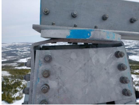
Figure 13: Bent Plate at Structure 2136 in 2021
