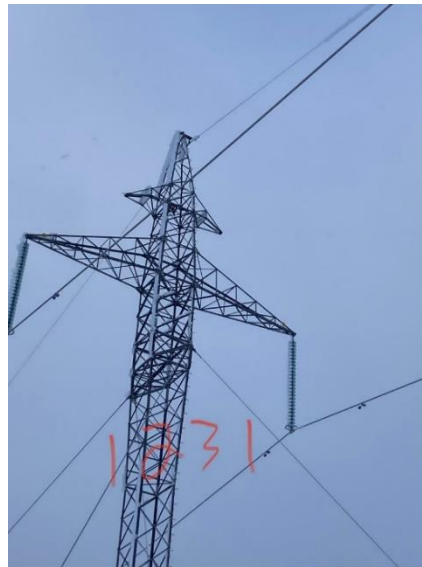
Figure 10: Ice on OPGW at Structure 1231 before Failure
