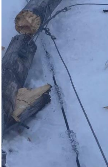
Figure 7: Distribution Line Failure from Freezing Rain in Red Bay
