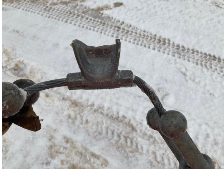
Figure 17: OPGW Stockbridge Damper Failure
