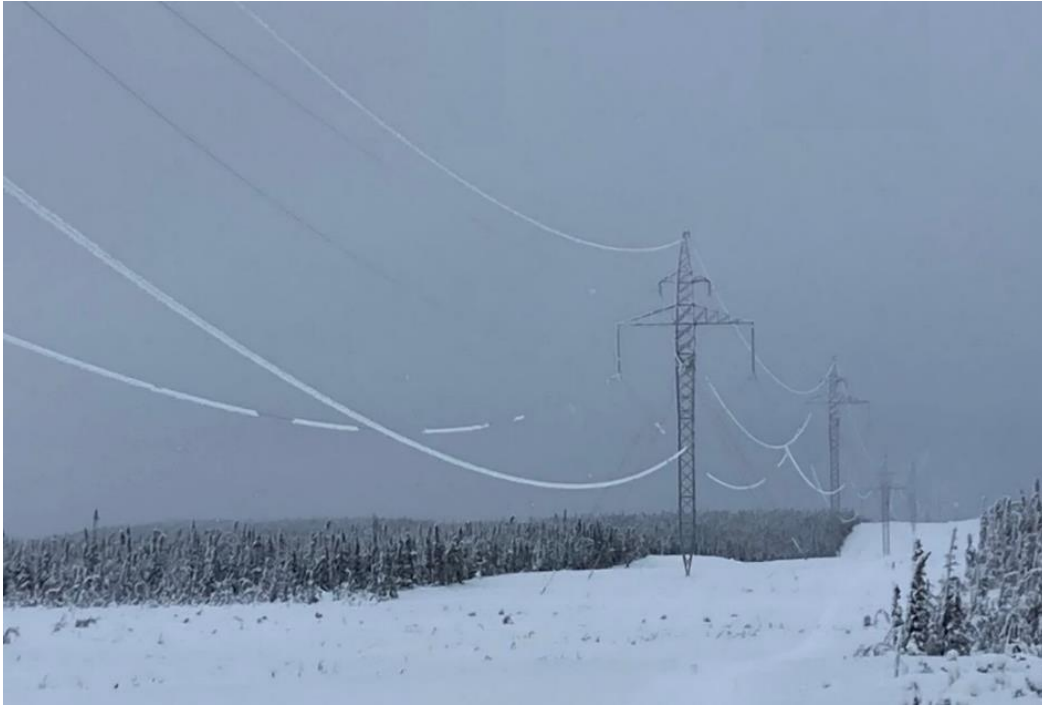
Figure 12: Ice Accumulation on Cables Immediately After Failure
