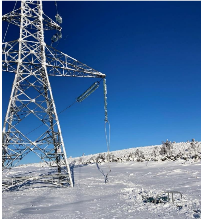
Figure 8: Failed Dead-End Assembly at Structure 1014
