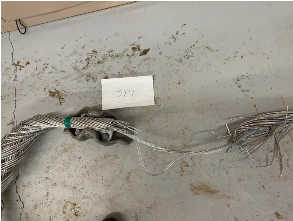
Figure 7: Structure 517 Broken Aluminum Strands
