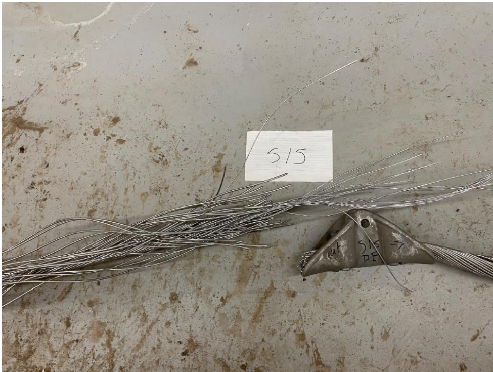
Figure 3: Broken EL2 at Structure 515
