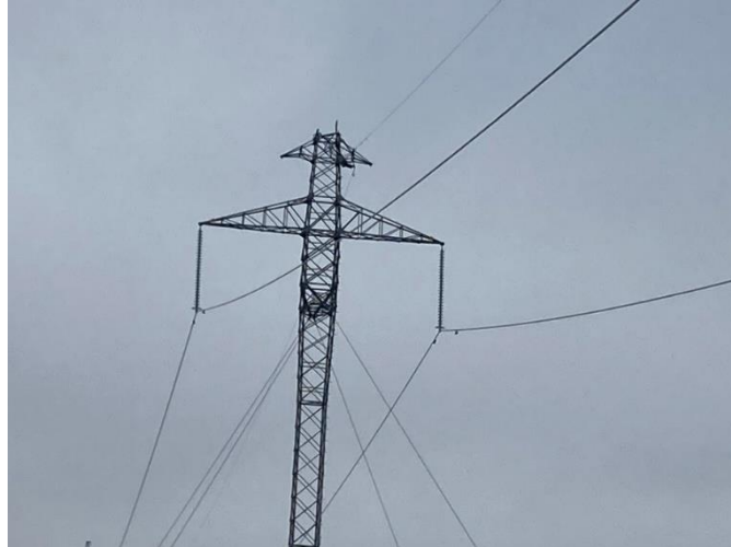
Figure 4: Failed OPGW Peak at Structure 1231
