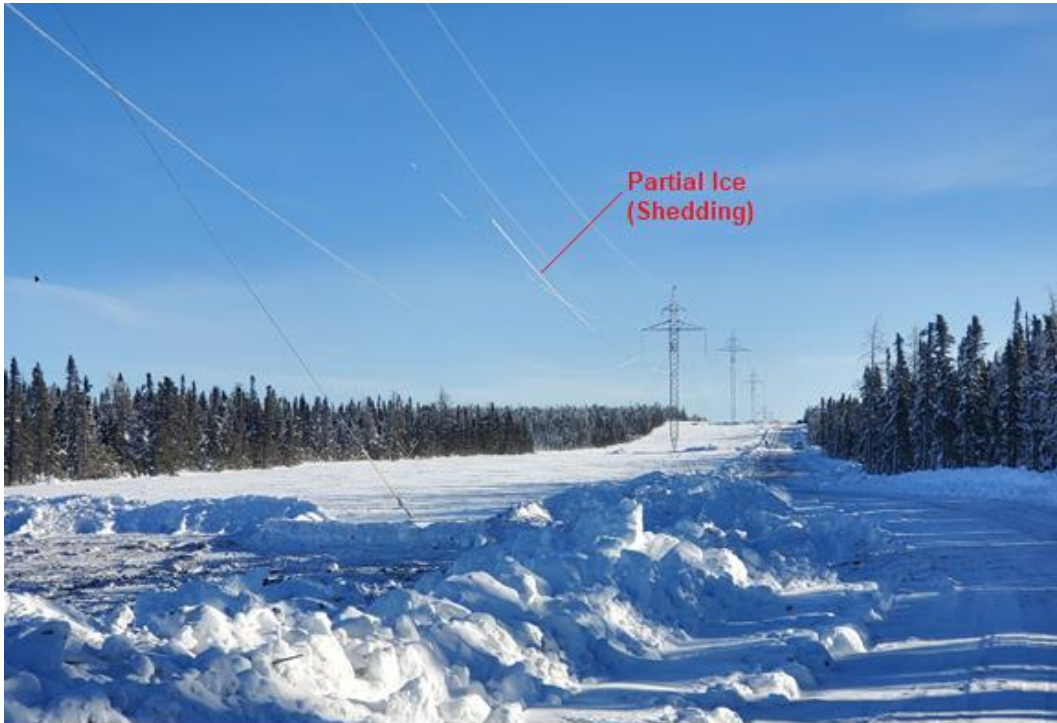
Figure 14: Cables with Partial Ice Accumulation (Indication of Ice Shedding)
