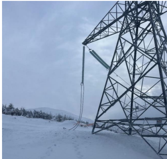
Figure 6: Failed Dead-End Assembly at Structure 1806
