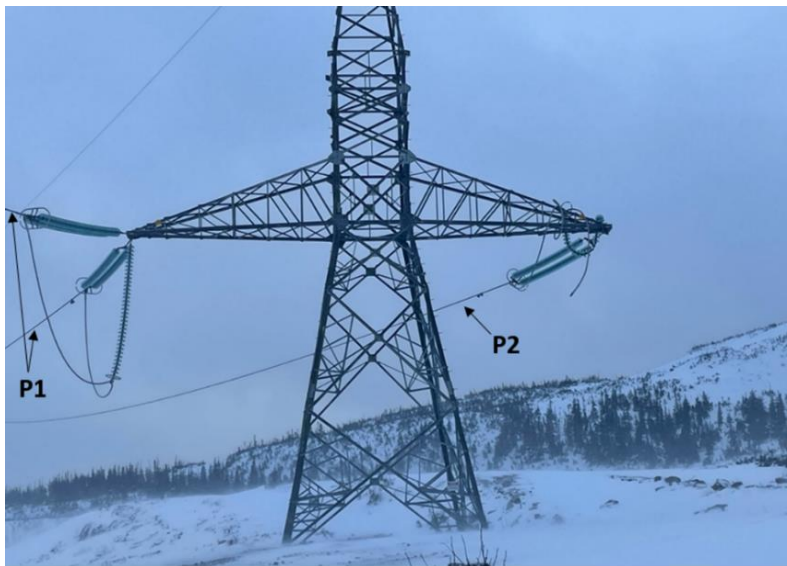
Figure 3: Structure 1872 with Failed Dead-End Assembly
