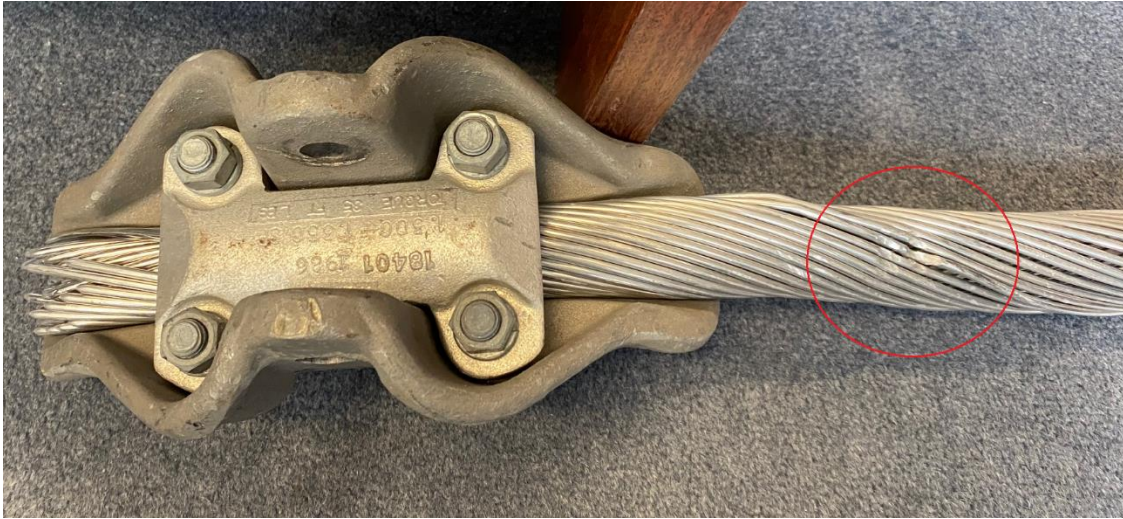
Figure 23: Dent in the Conductor near the Tangent Assembly from Structure 515
