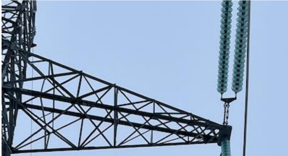
Figure 17: Dead-End Assembly with Newly Installed Safety Chain
