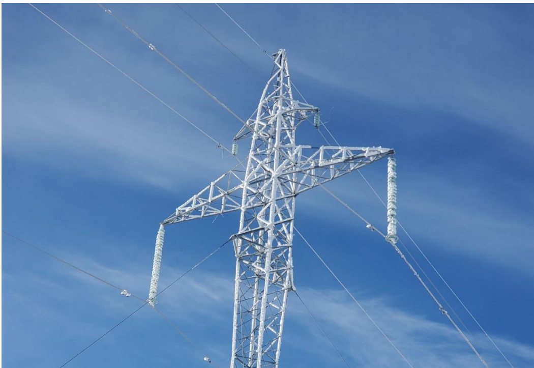
Figure 13: Ice Accumulation on Towers/Insulators (Mixture of Snow/Ice)
