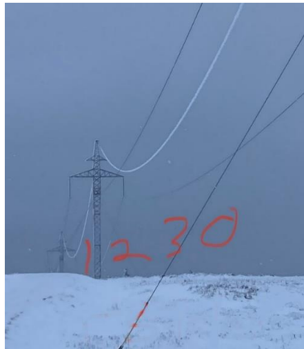
Figure 9: Ice on OPGW at Structure 1230 before Failure
