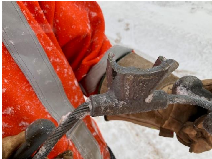
Figure 18: OPGW Stockbridge Damper Failure
