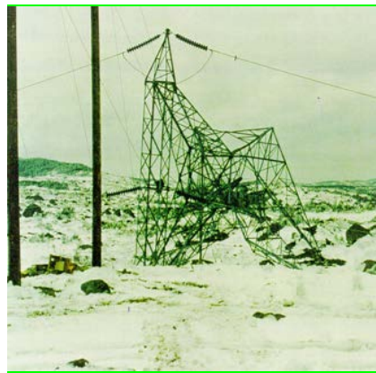
35 36 Figure 1.2 Large Angle Tower Failure near Hawke Hill (1988 Storm Avalon Peninsula, Haldar, 1996) 37
