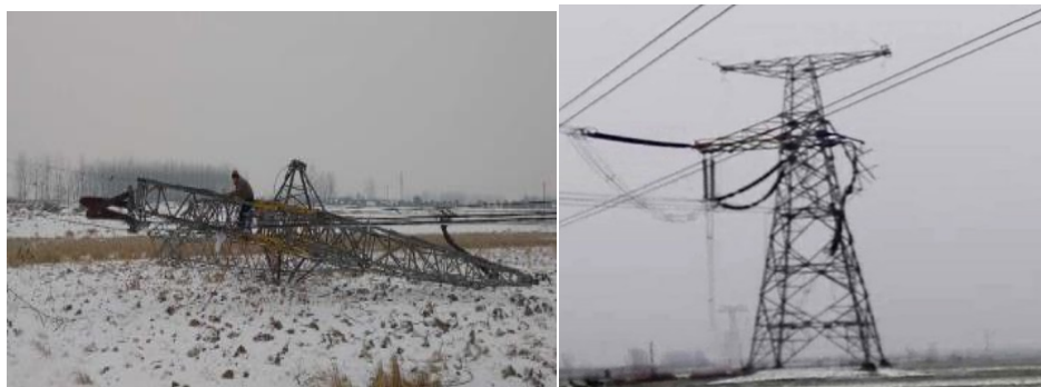
2322 2323 Figure 8.8a Photo of the collapsed tower and (b) Tower’s cross arm failure (Liu, 2021)
