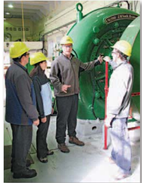
The Petty Harbour plant, commissioned in 1900 as Newfoundland's first hydroelectric plant, received a $1.8 million overhaul in 2006.
