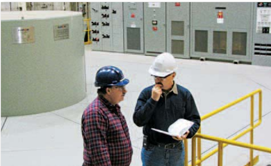
In central Newfoundland, Fortis Generation holds a 51 per cent interest in the Exploits River Hydro Partnership.
