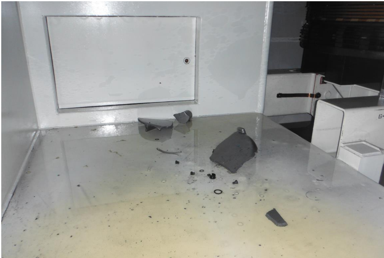
Picture – Below the Tap Changer on the shelf in the Transformer.
