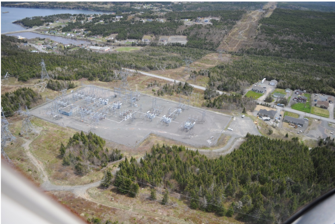
Western Avalon Terminal Station
