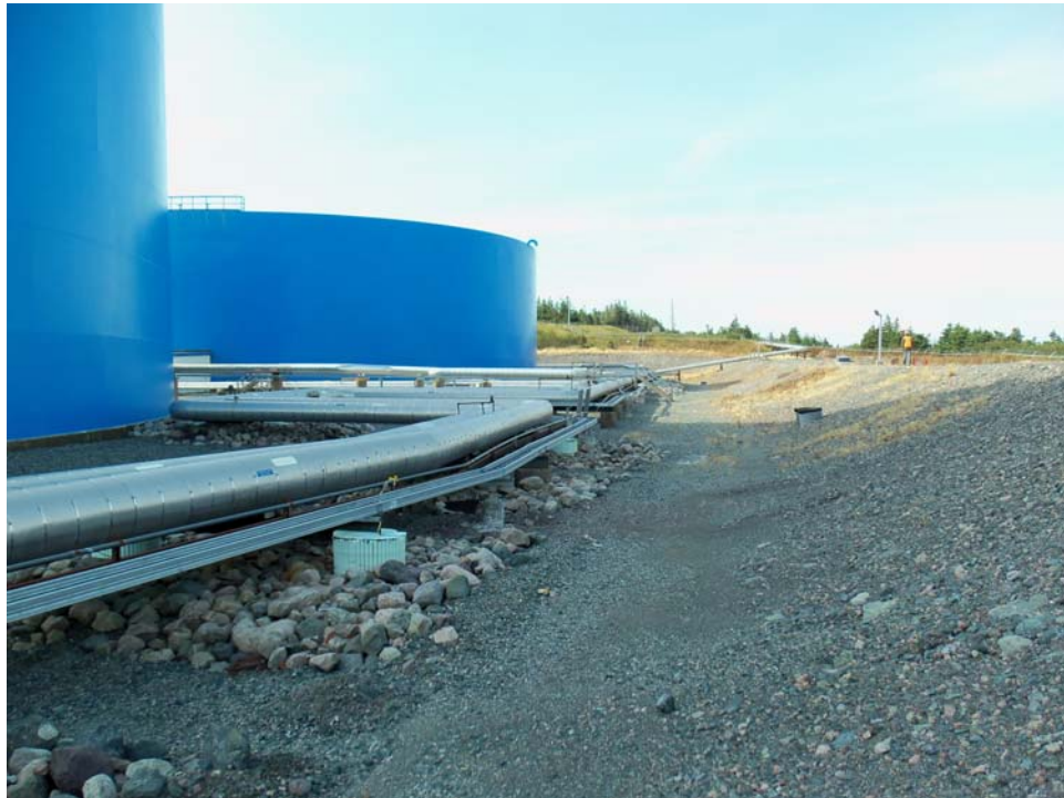
Figure 2: Tanks 3 and 4 and the berm to the left which must be ascended to access those two tanks.
