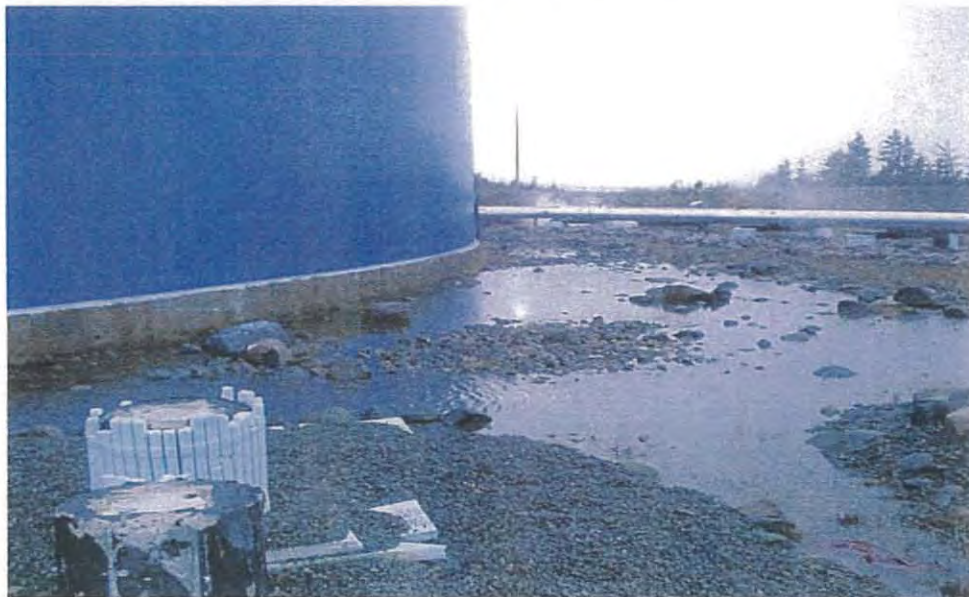
Figure No.8 Water In Compound On West Side
