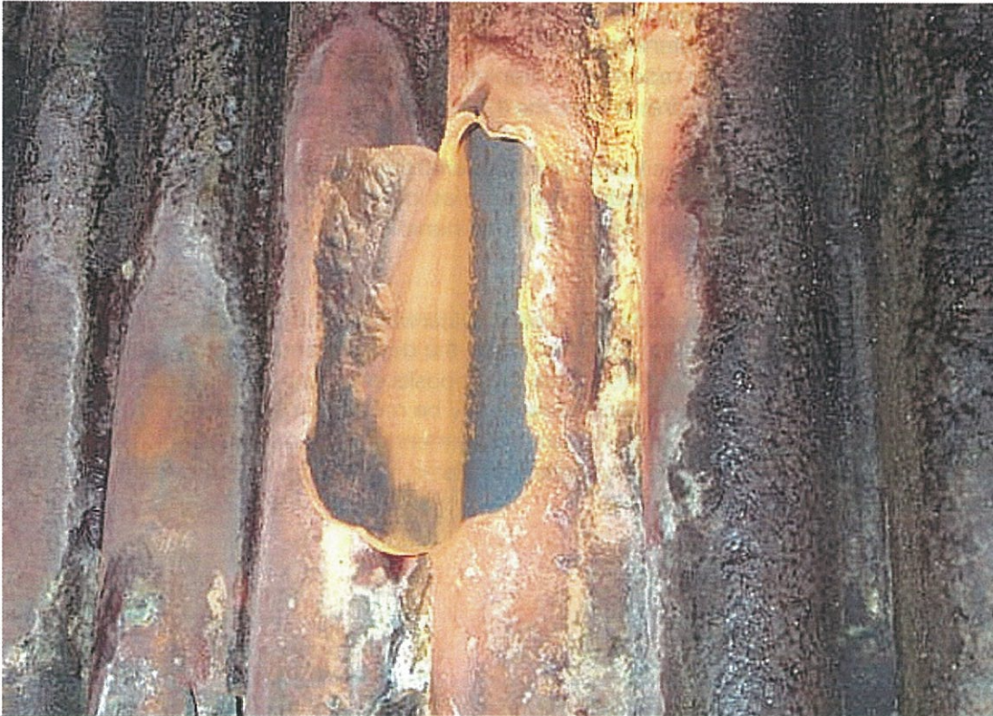
Figure 1. Original tube failure - Tube 56 from D corner 53' elevation
