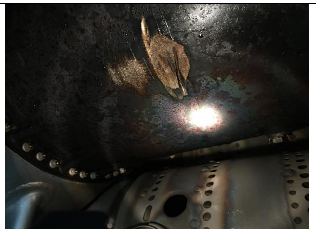
Turbine support housing holed & fretted
