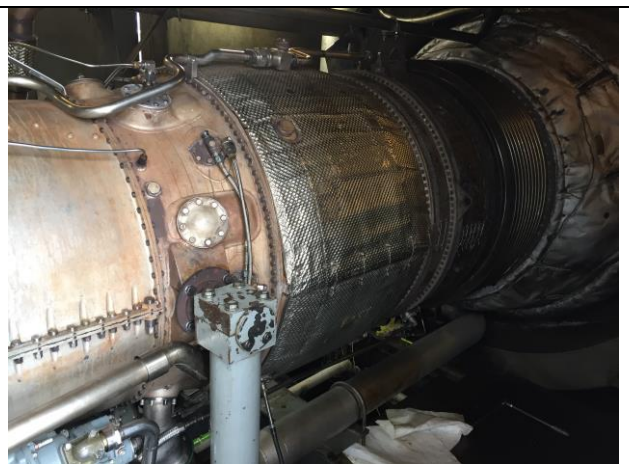
Gas Turbine 202040 installed
