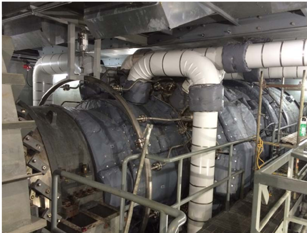
Figure 3: Holyrood Siemens Combustion Turbine
