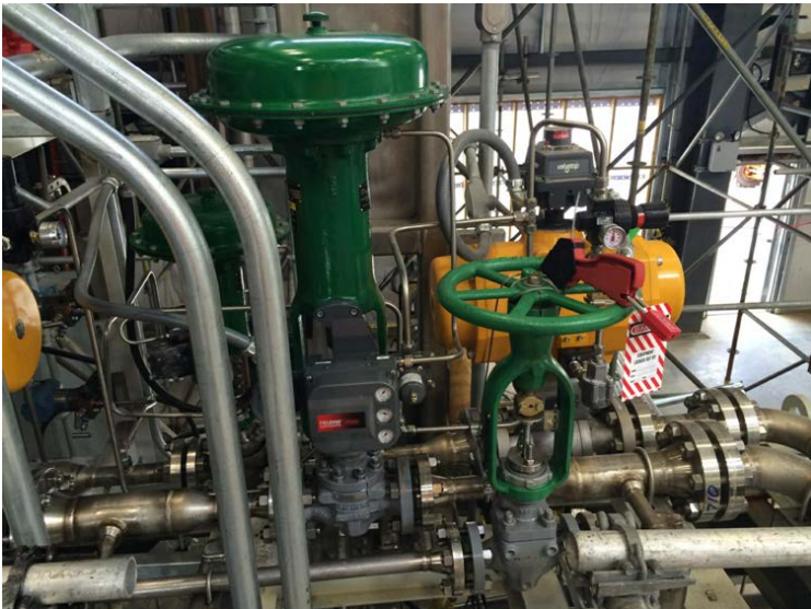
Photo 2: Fuel bypass valve locked and tagged
