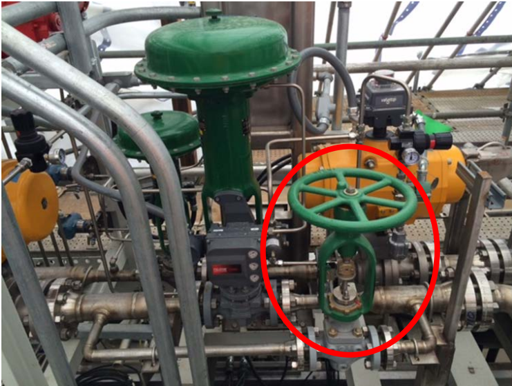
Photo 1: Fuel bypass valve
