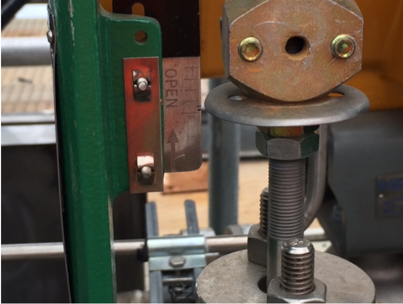
Photo 3: Close up of fuel bypass valve position indicator
