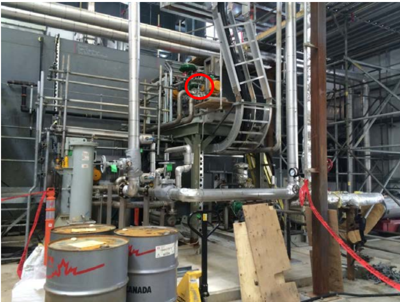
Photo 4: Fuel bypass valve location within the plant
