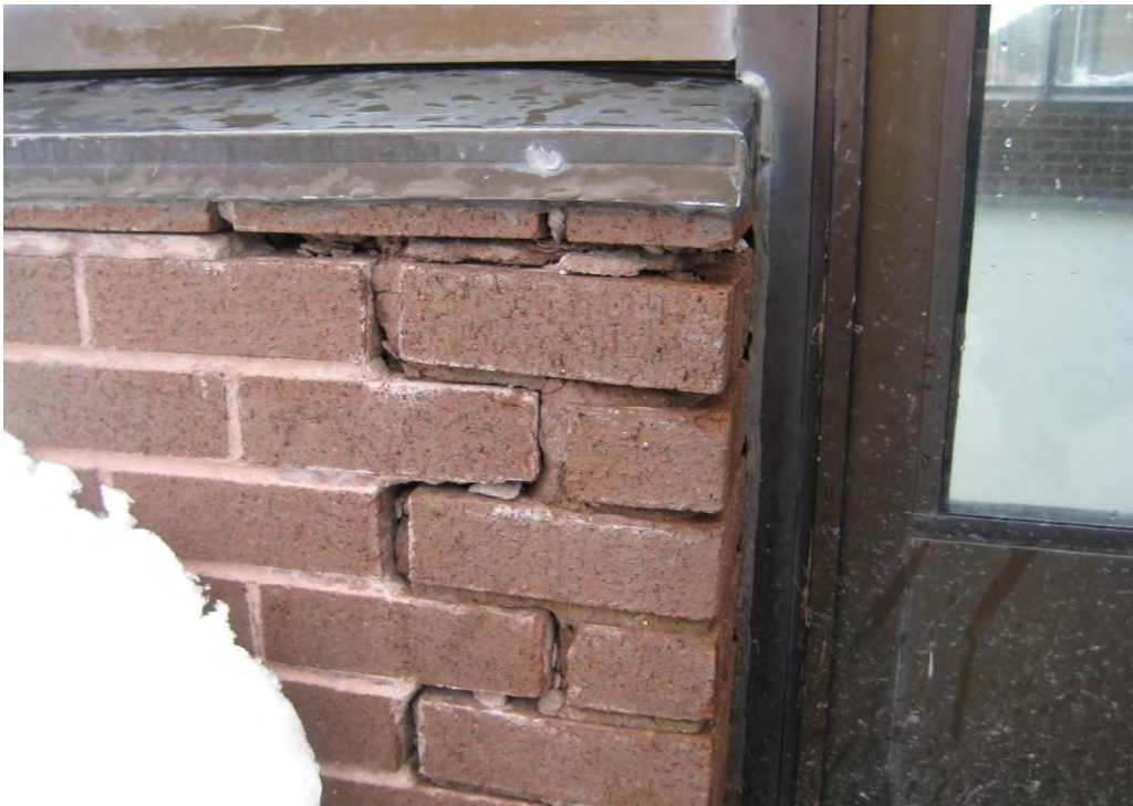
Figure 5 - Cracked Exterior Block (2009)
