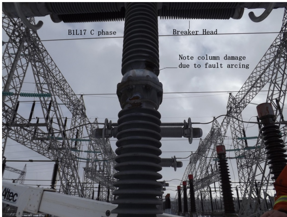
Figure 2-5d: B1L17 Vertical Column Arcing Damage
