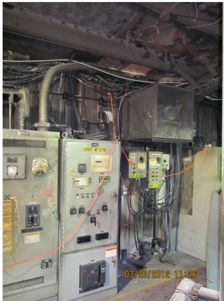
Figure 3: Switchgear after the Fire
