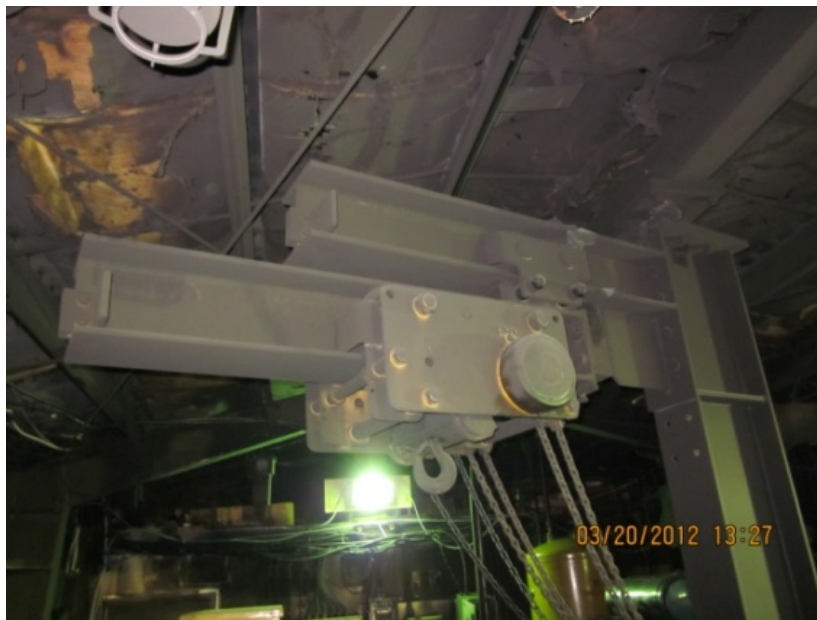
Figure 2: Jib Crane after the Fire
