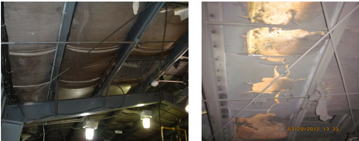
Figure 4: Building Insulation Before and After the Fire (left to right)
