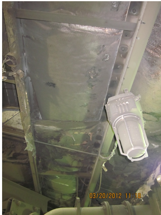
Figure 7: Fire Damage to Engine Hall Ceiling
