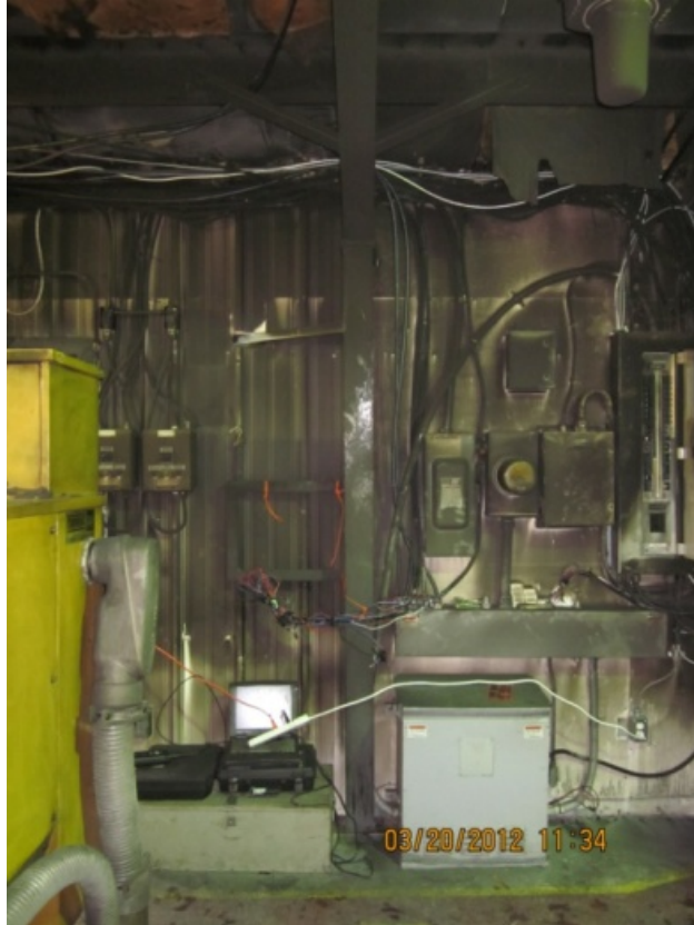
Figure 1: Station Service Equipment after the Fire
