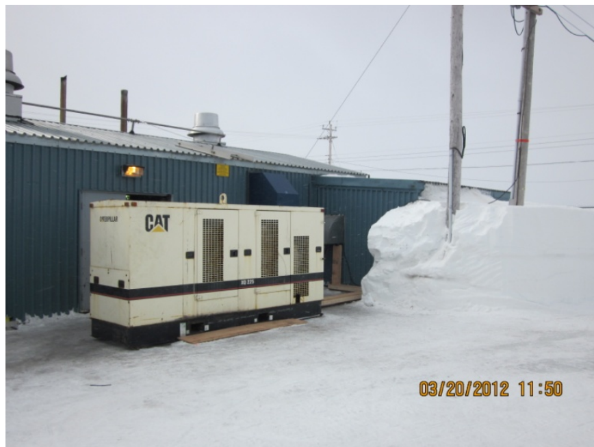
Figure 9: 225 kW Mobile Genset Installation
