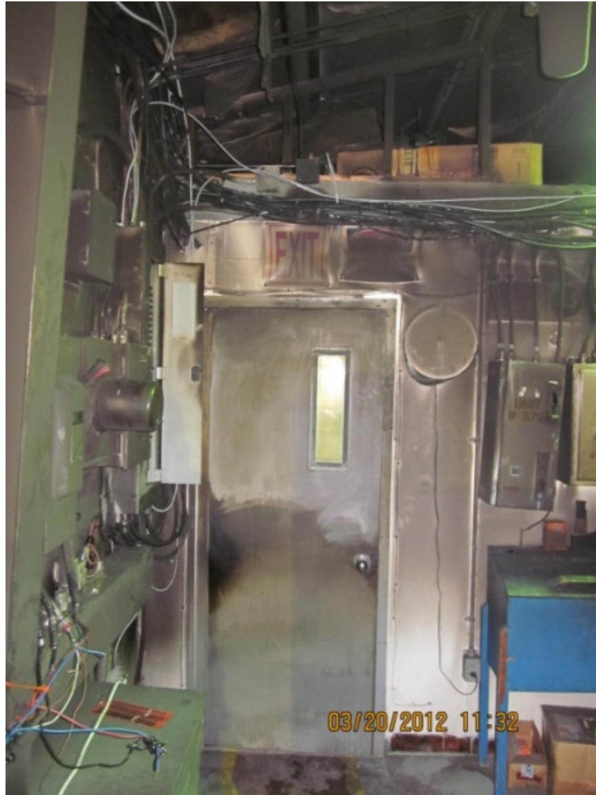
Figure 5: Fire Damage to Door, Wiring, Walls and Ceiling
