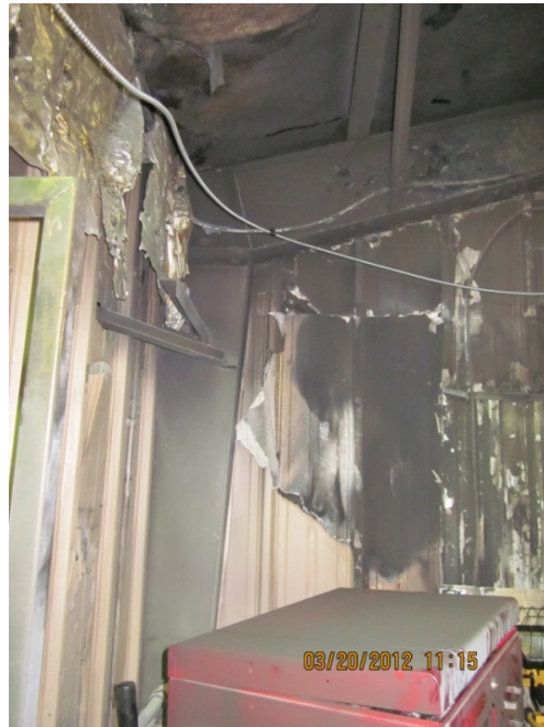
Figure 8: Fire Damage to Interior Panelling
