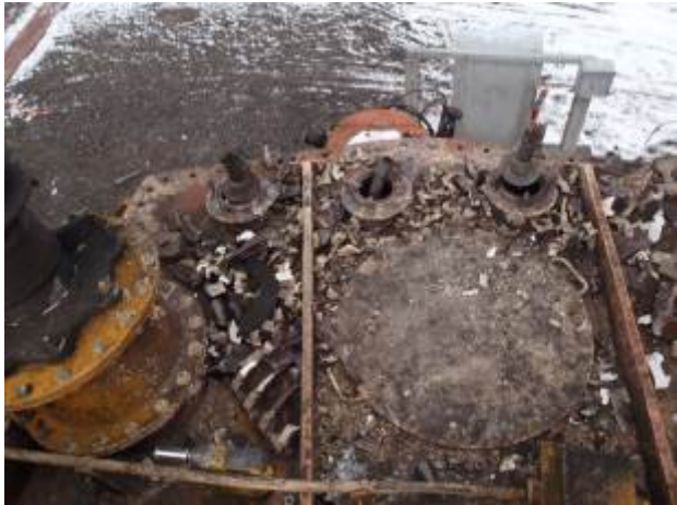
Photo 3 – Cover Open & Broken Bolts
