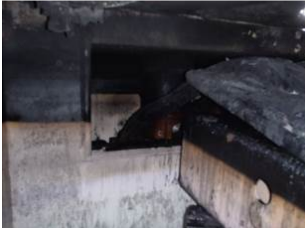
Photo 13 – Fire Line on Tank Wall & Core Clamp
