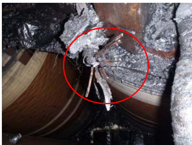
Photo 19 – LV2 Winding Lead Broken
