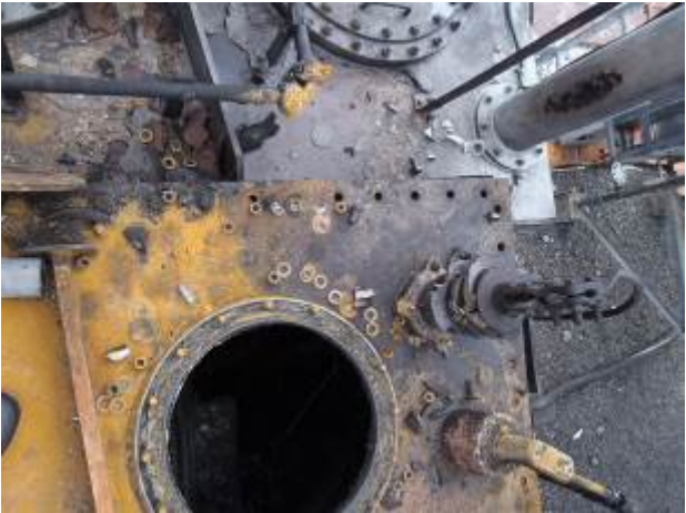
Photo 4 – Cover Open & Broken Bolts
