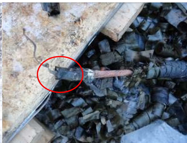
Photo 20 – LV2 Bushing Lead Broken at the Crimp
