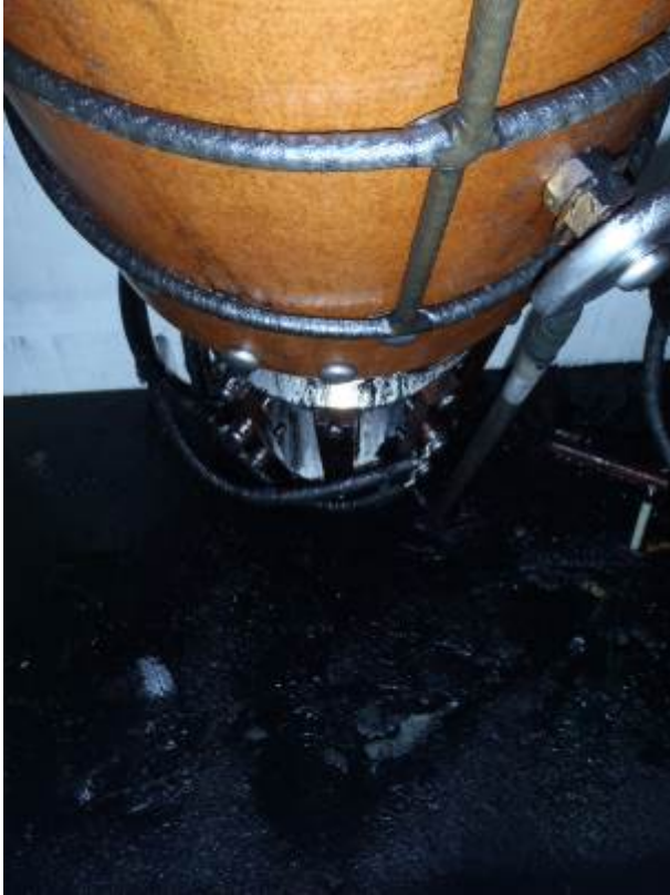
Photo 11 – LTC Compartment (Phase 3)
