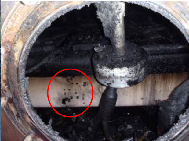
Photo 16 – LV1 Bushing & Flashover marks
