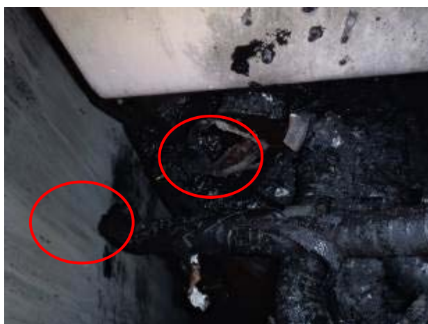
Photo 21 – LV1 Winding Lead Broken
