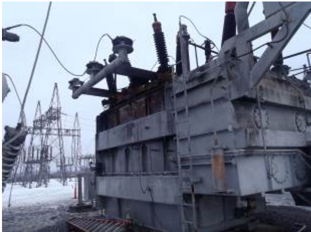
Photo 1 – Cover Open & Broken Bolts
