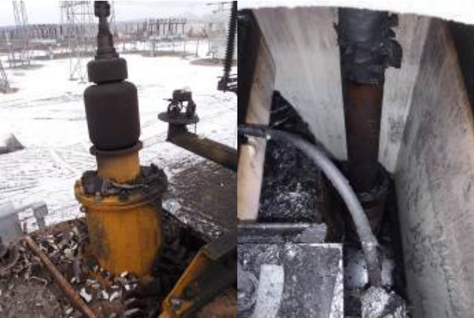
Photo 8 – HV1 Bushing Porcelain
