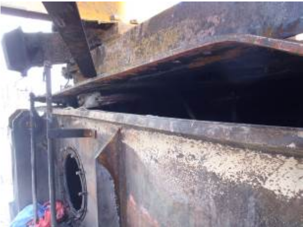
Photo 2 – Cover Open & Broken Bolts
