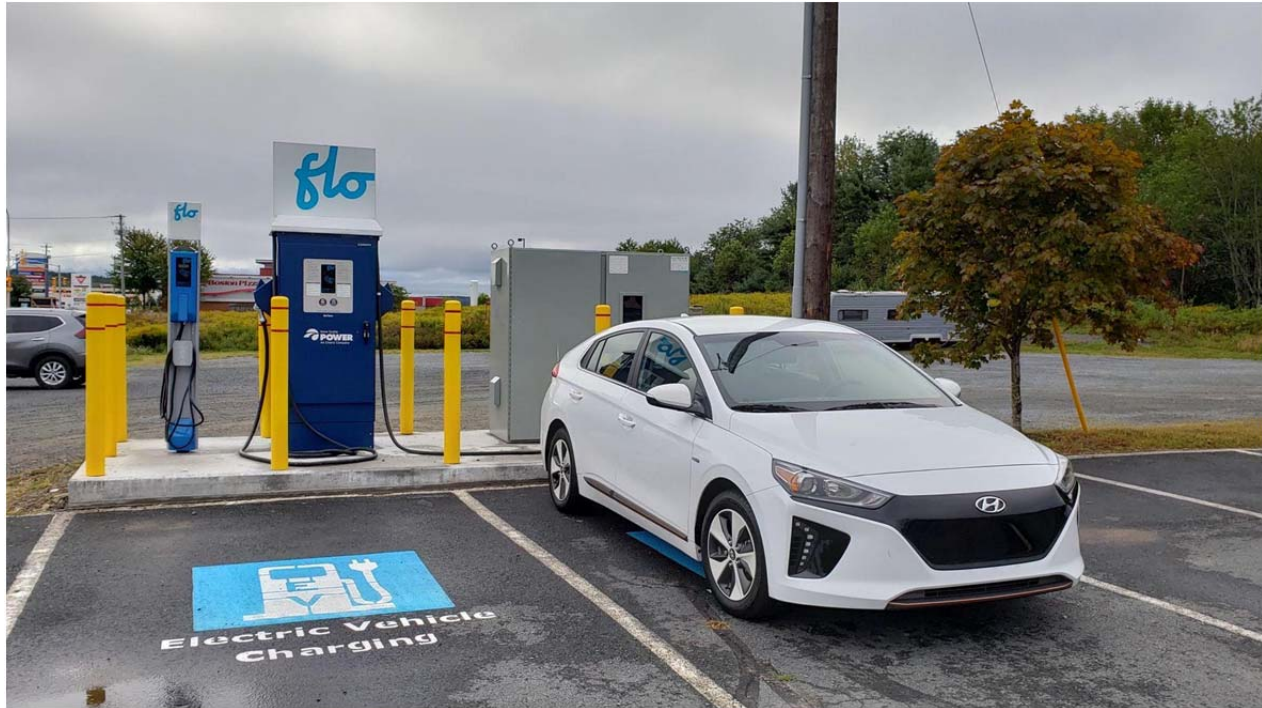
Example of EV Charging Station installed by Nova Scotia Power
