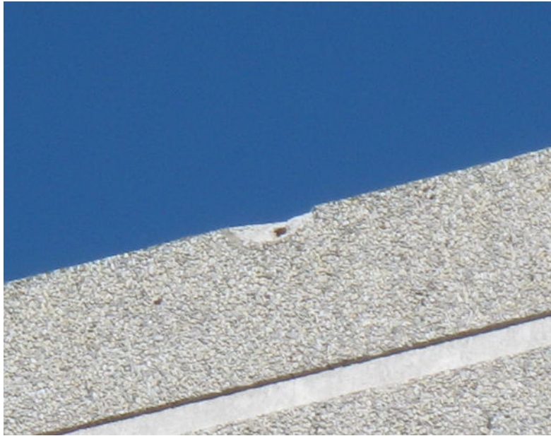
Photo 1: Spall at top of panel.
