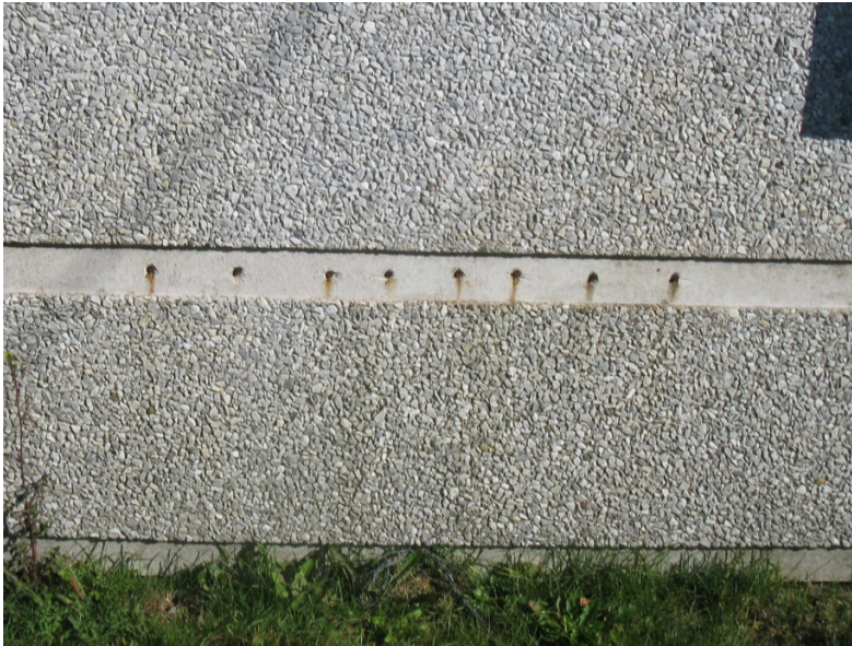
Photo 15: Rust at exposed anchors.
