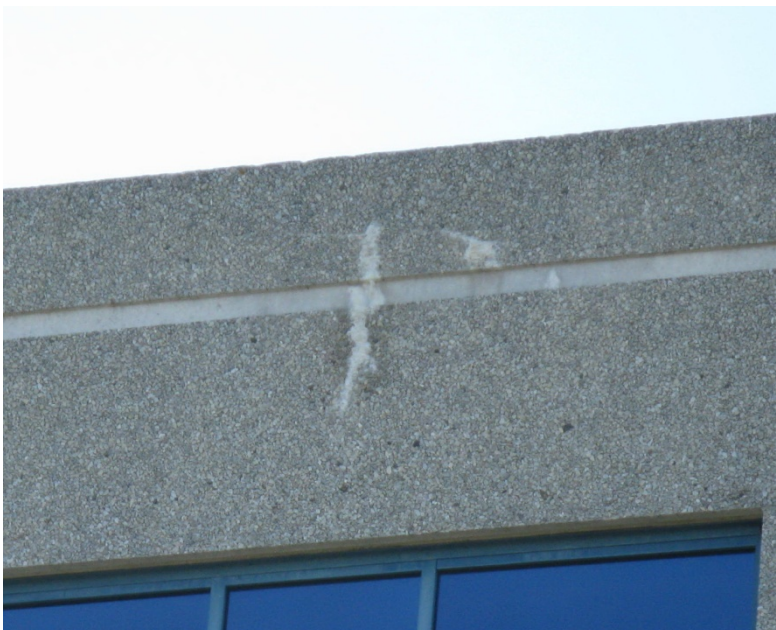
Photo 4: Minor cracks and efflorescence crystal formation.
