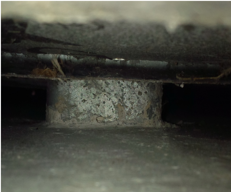
Photo 24: Hollow structural steel panel support.
