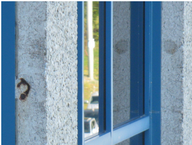
Photo 6: Exposed end of reinforcing/lift anchor and typical mortar repair beyond.
