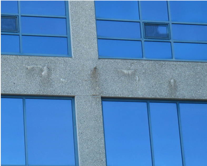
Photo 3: Minor cracks and efflorescence crystal formation.
