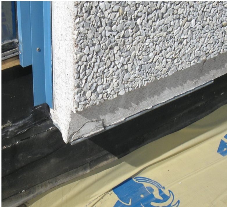
Photo 28: Galvanized steel angle at panel bottom.
