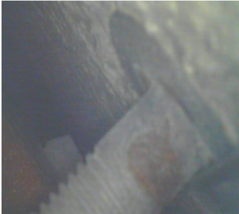
Photo 27: Large diameter panel support bolt.
