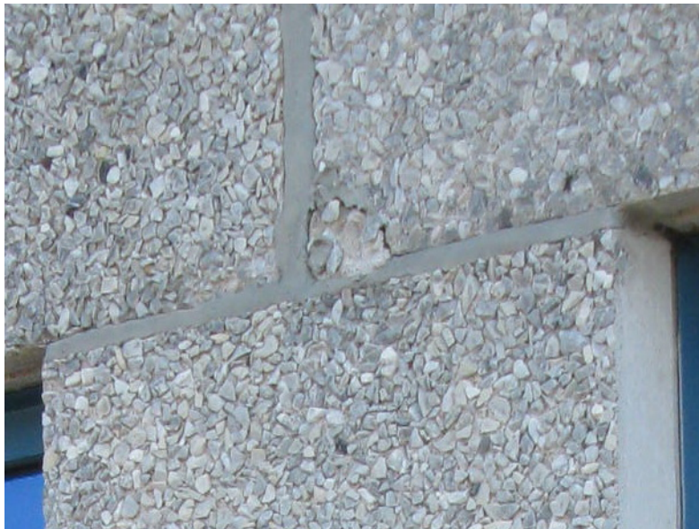
Photo 2: Spall and repair at lower left corner of panel.
