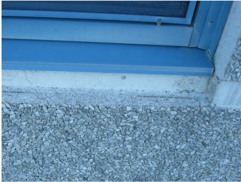
Photo 5: Minor cracks in panel.
