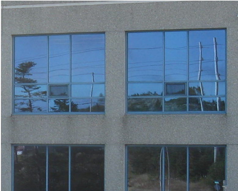
Photo 13: Water runoff stains adjacent to windows.
