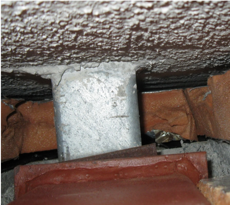
Photo 23: Hollow structural steel panel support.
