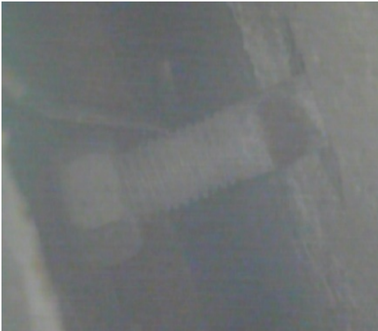
Photo 26: Large diameter panel support bolt.
