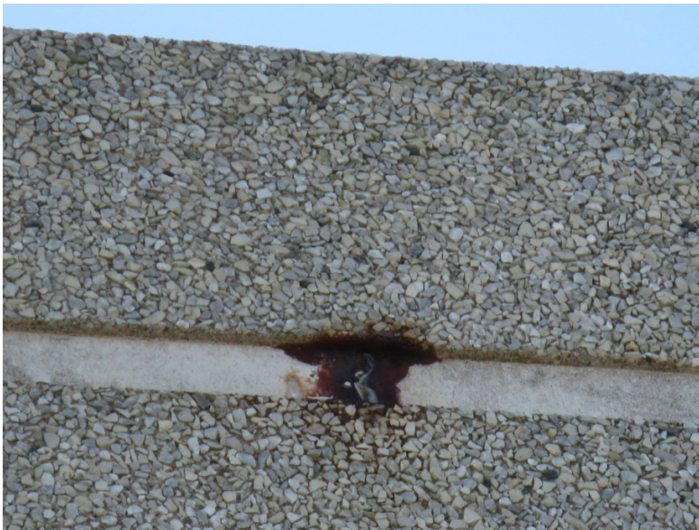
Photo 8: Exposed end of steel section.
