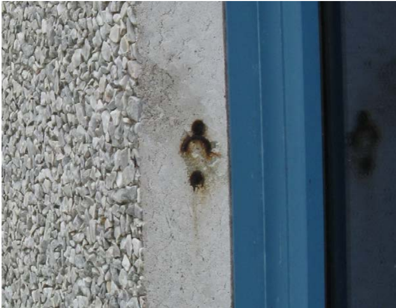
Photo 7: Exposed end of reinforcing/lift anchor.
