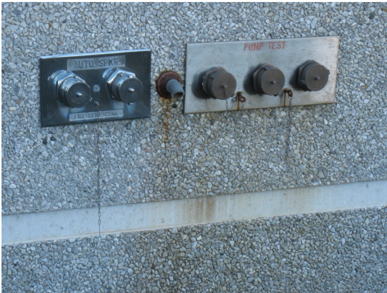
Photo 14: Stains/rust around building service equipment.
