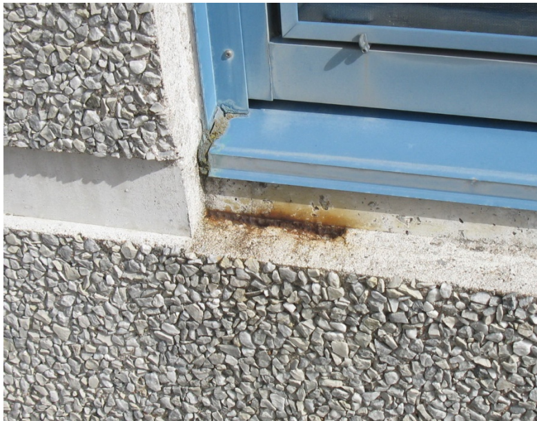
Photo 9: Exposed steel rebar reinforcing.
