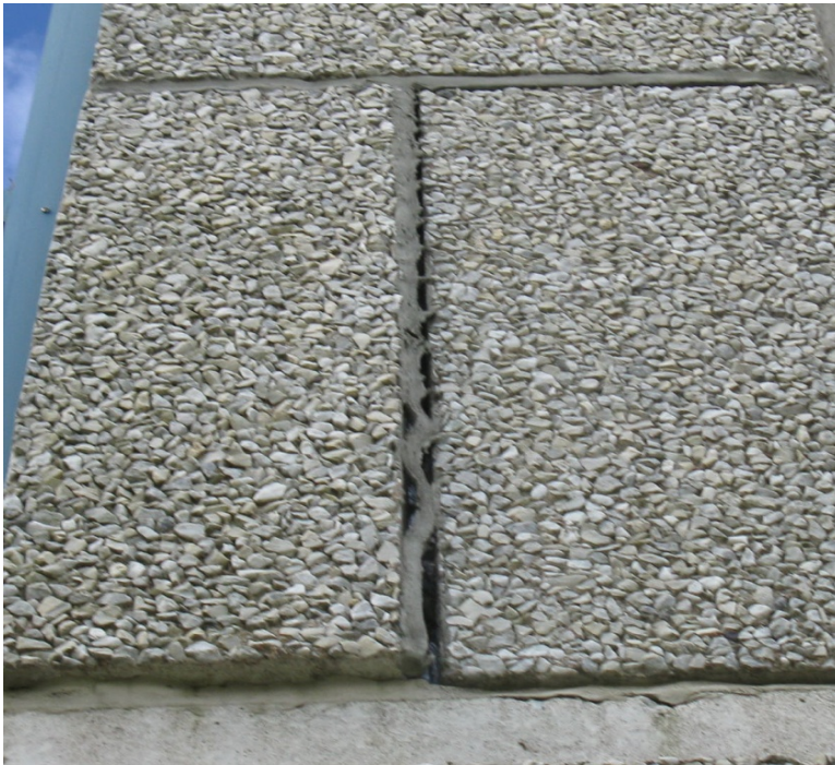
Photo 22: Sealant detached on both sides of joint.
