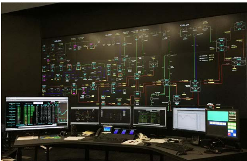
Figure 4: ECC One Line Display (Post Upgrade)
