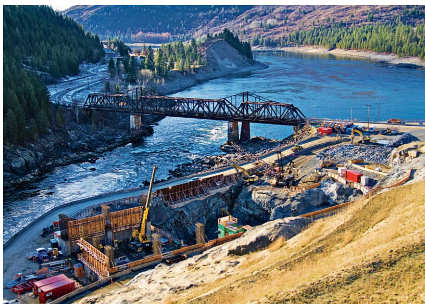
Construction of the $900 million 335-MW Waneta Expansion hydroelectric generating facility is progressing well.
