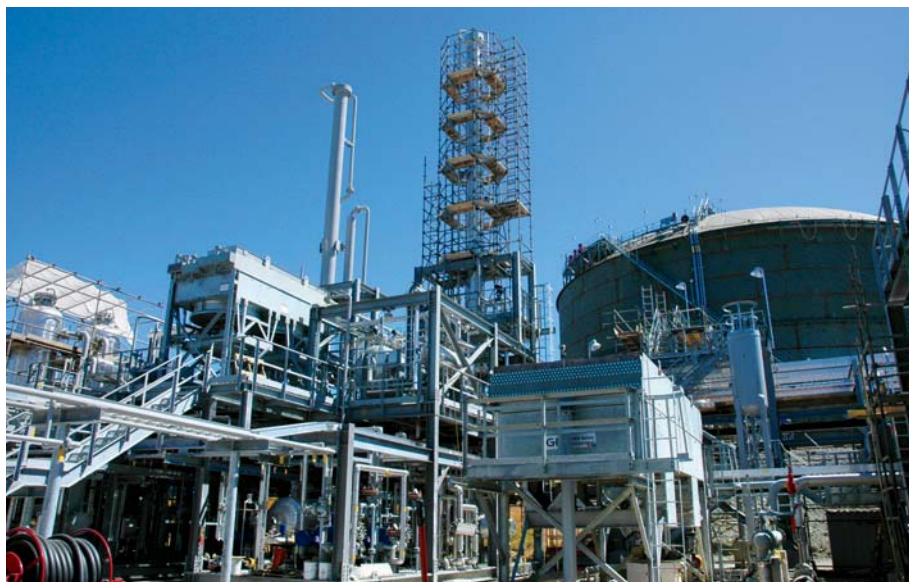
Construction of the $210 million Terasen Gas (Vancouver Island) liquefied natural gas storage facility is nearing completion.
