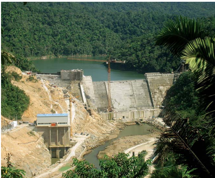
The US$53 million 19-MW Vaca hydroelectric generating facility on the Macal River in Belize will be commissioned in March 2010.
