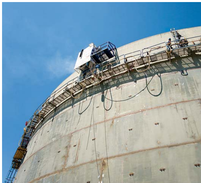
The Terasen Gas (Vancouver Island) liquefied natural gas storage facility is scheduled to come into service in 2011.
