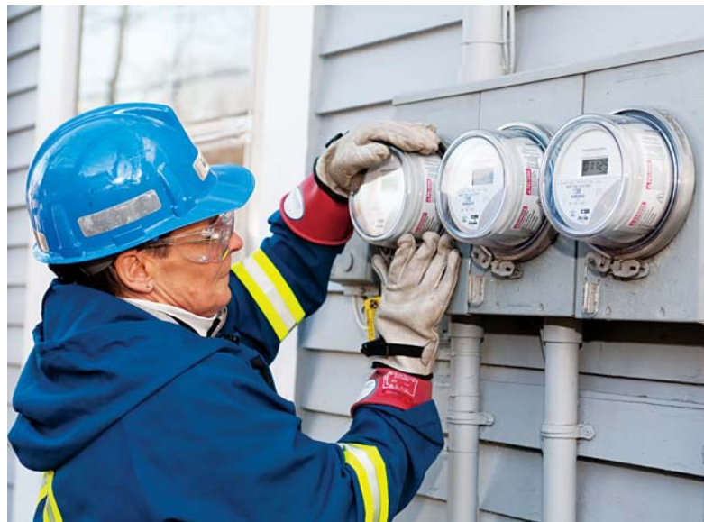
Maritime Electric serves approximately 74,000 customers on Prince Edward Island.
