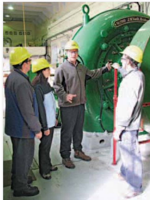
The Petty Harbour plant, commissioned in 1900 as Newfoundland's first hydroelectric plant, received a $1.8 million overhaul in 2006.
