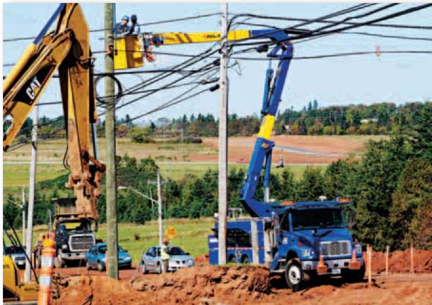
Maritime Electric is the principal electric utility on Prince Edward Island, serving approximately 71,000 customers, or 90 per cent of electricity consumers in the Province.
