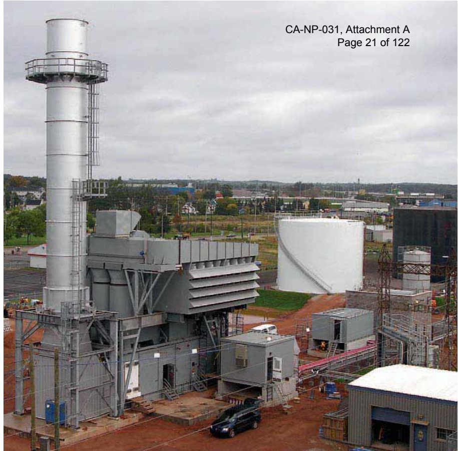
Maritime Electric's new 50-MW combustion turbine generator will provide increased reliability and security of energy supply on Prince Edward Island.
