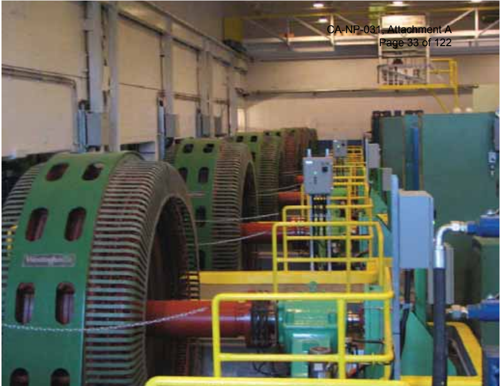
In central Newfoundland, Fortis Generation holds a 51 per cent interest in the Exploits River Hydro Partnership.
